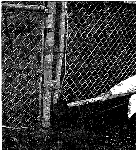
Weld on fence gate broke when pulled
