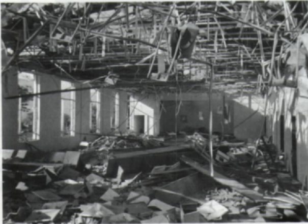
January 23, 1994—Medellin, Colombia: Interior window and structural damage caused by the bombing of the Mormon chapel in Medellin.
