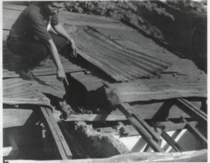
February 1, 1994—Manila, Philippines: Aftermath of the bombing of the Caltex building. The Alex Boncayao Brigade claimed credit for the attack.
