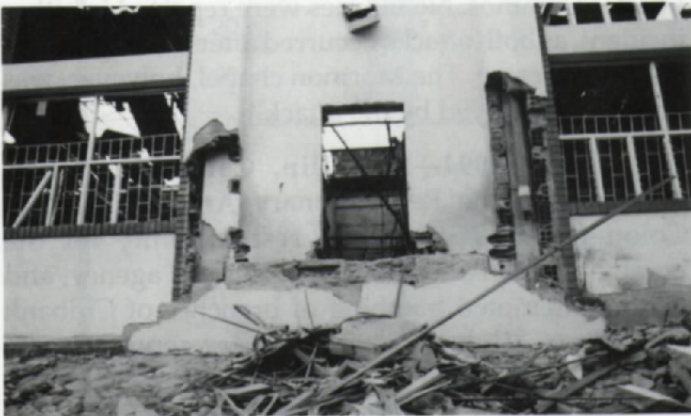
January 23, 1994—Bucaramanga, Colombia: Damage to a Mormon chapel in Bucaramanga caused by a bomb planted by suspected Marxist guerrillas.
