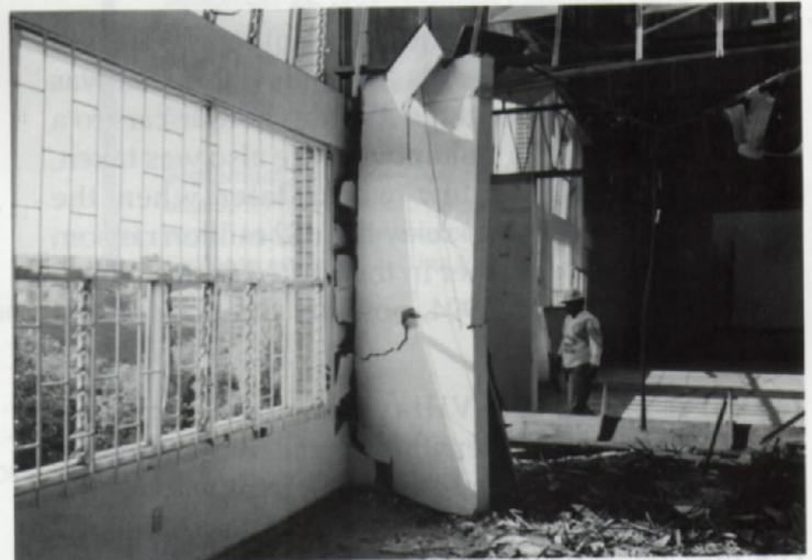
January 23, 1994—Bucaramanga, Colombia: View of interior damage to the Bucaramanga Mormon chapel.
