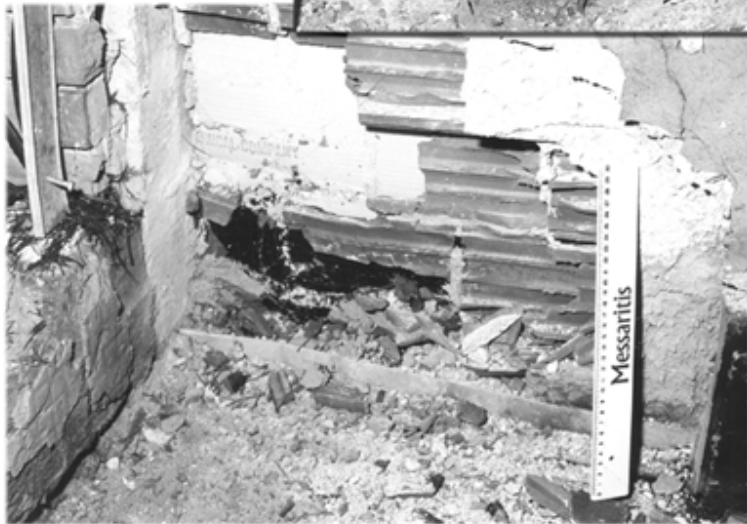
February 3, 1998—Athens Greece: Pictured is the bomb damage done to a McDonalds restaurant in the Vrillissia suburb of Athens
