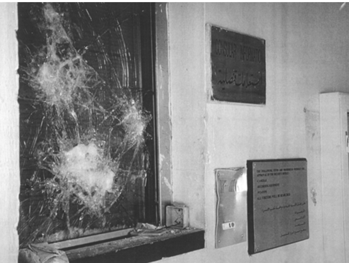
December 19, 1998, Damascus, Syria. Damage to the Consular section intake window and intercom.
