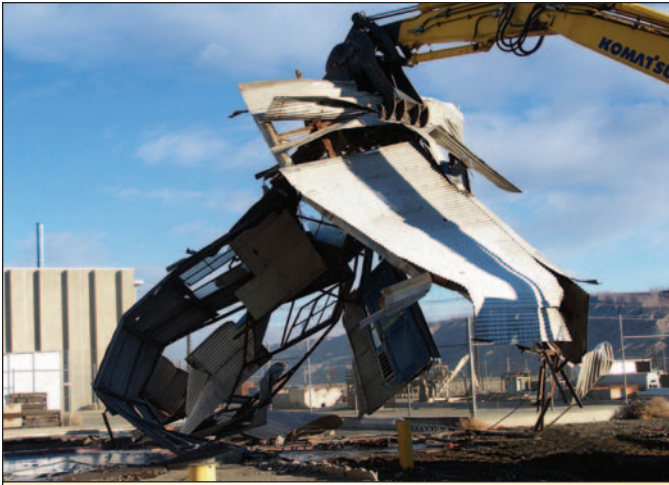
Radioactive Facility Demolition: The demolition of the decontaminated 334A Waste Acid Storage Building at the Hanford Reservation at Richland, Washington.
