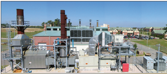
Integrated Energy System: An Integrated Energy system installed at the Fort Bragg 82nd Airborne Central Heating Plant.
