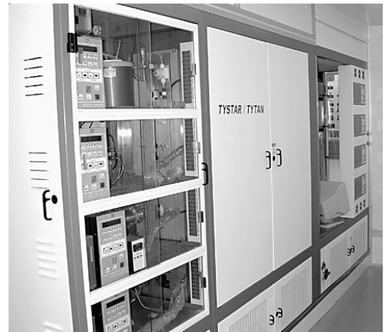
Computer-controlled research tube furnaces for growth of SiO 2 , Si 3 N 4 , and other CVD materials.
