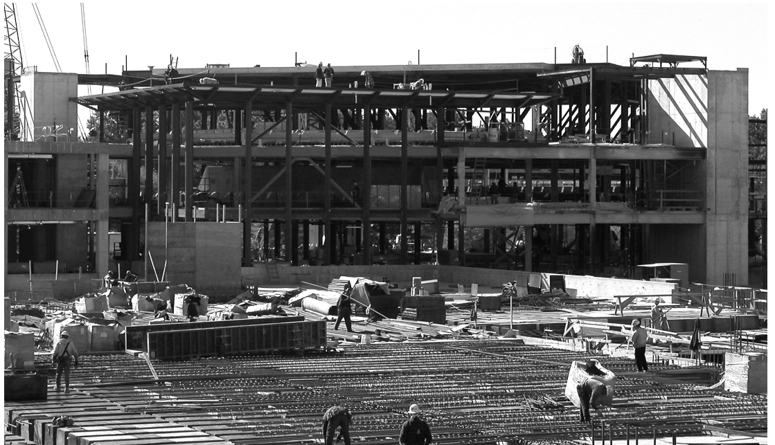
Construction of the Advanced Measurement Laboratory Cleanroom as seen in late October 2001.
