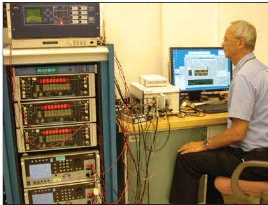
PMUs – a key component of electric power grid modernization. The figure shows the NIST Calibration System for PMUs. The PMUs are the two instruments on top of the cabinet.
