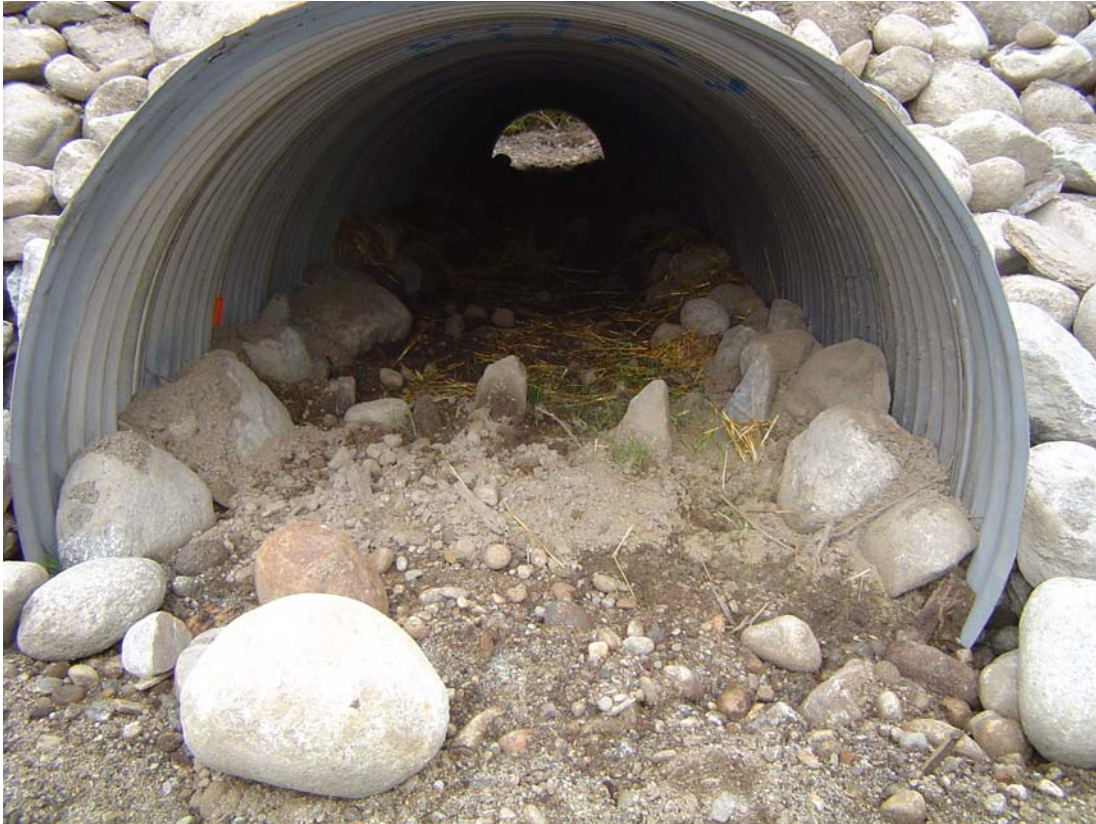
Photo 2. Culvert inlet at Road 6256 MP 3.244. Dry Channel, note the rock weirs, channel banks and rip rap.
