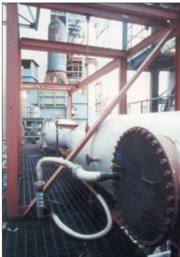
The sorbent injection into the duct upstream of SO x -NO x -Rox Box™ system.
