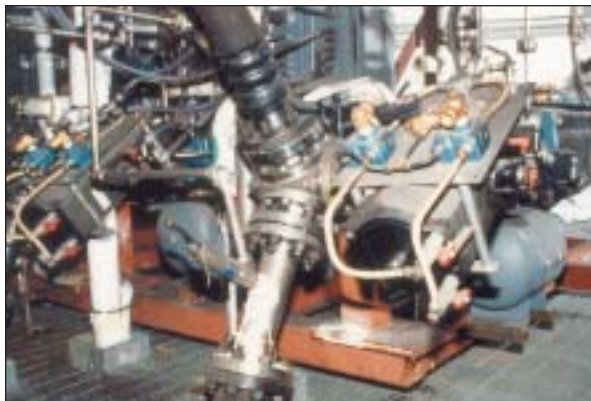
The coal slurry and sorbent injectors for the Tidd PFBC demonstration.
