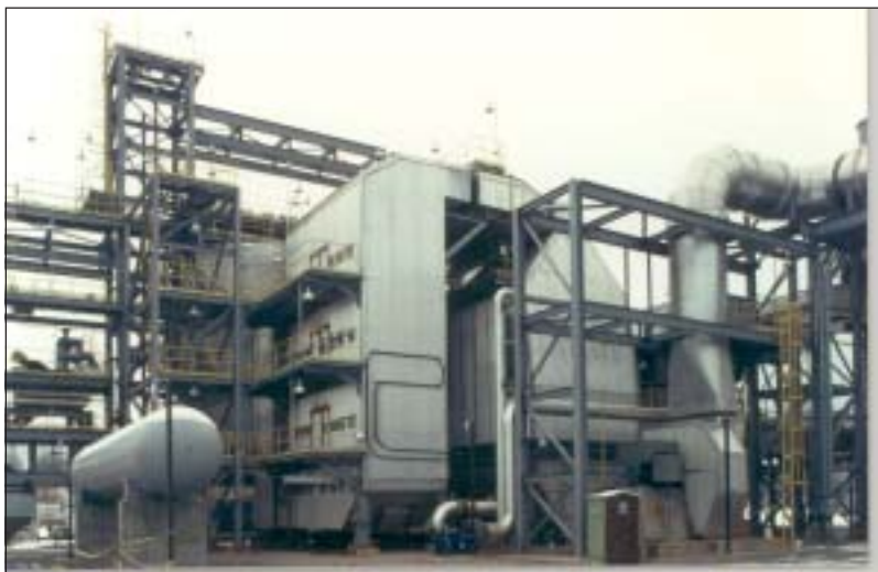
The SNOX™ demonstration at Ohio Edison's Niles Station Unit No. 2 achieved SO 2 removal efficiencies exceeding 95% and NO x reduction effectiveness averaging 94%. Ohio Edison is retaining the SNOX™ technology as part of its environmental control system.
