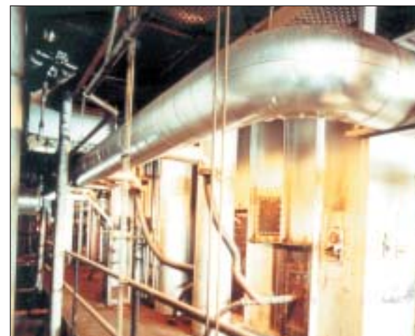
The sorbent injection system for the GR-SI technology.
