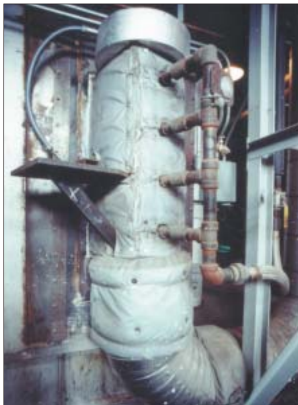
The natural gas injector was installed on the corner of Hennepin Station's tangentially fired boiler.
