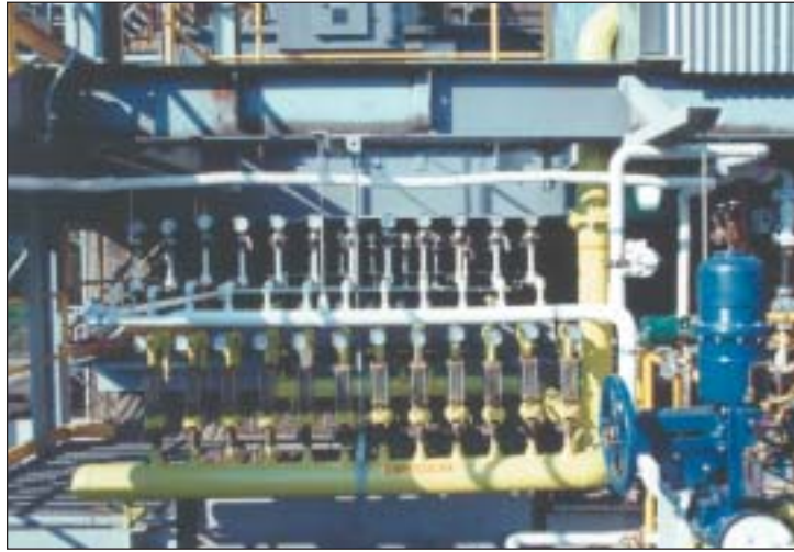
CZD/FGD lime slurry injector control system.
