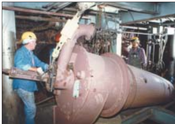
NO_x emissions at Georgia Power's Plant Hammond were reduced by 63 percent with Foster Wheeler's low- NO_x burners, shown here, and advanced overfire air.
