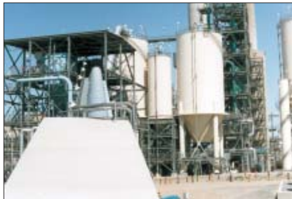
The Piñon Pine coal conveyor from storage dome to the plant.
