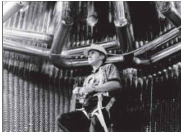
Inside the Texaco gasifier.
