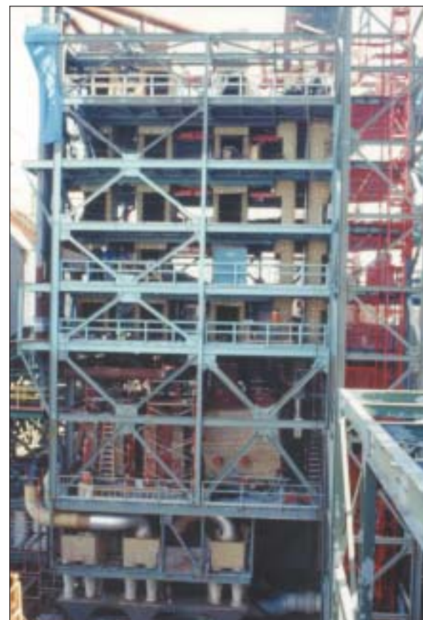
Eight SCR catalysts with various shapes and compositions were evaluated side by side at Gulf Power's Plant Crist using high-sulfur coal. NO x reductions of 80 percent were achieved.
