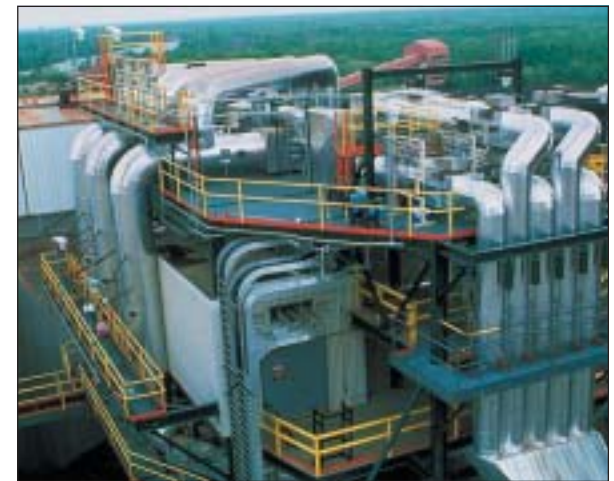
The SCR demonstration facility at Southern Company's Plant Crist.
