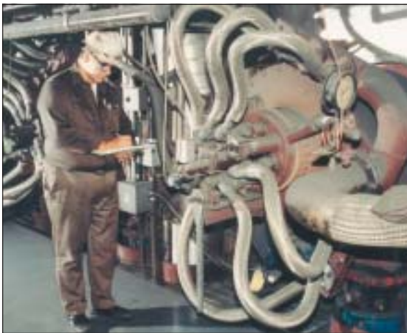
Foster Wheeler's LNBs used at Cherokee Station for the GR-LNB demonstration.
