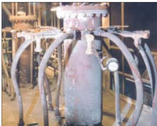
LIMB furnace sorbent injection lines
