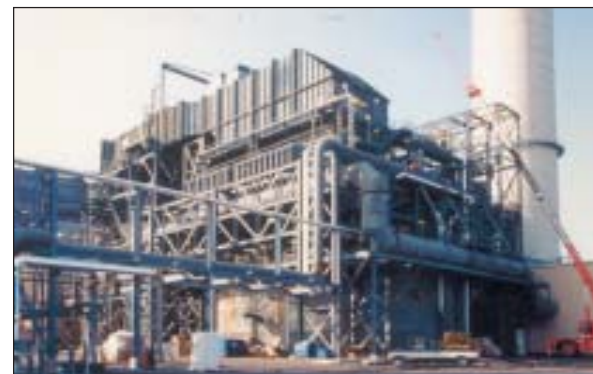
Pure Air on the Lake L.P. demonstrated an FGD process that removed 95 percent or more of SO 2 emissions at the Bailly Generating Station in Indiana.
