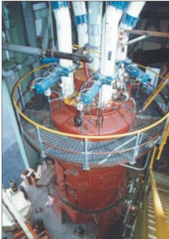
The coal pulverizer is part of Babcock & Wilcox Coal Reburning. This system has been retained by Wisconsin Power and Light for NO x emission control at the Nelson Dewey Station.
