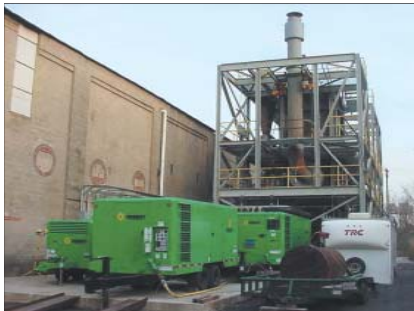
ThermoChem's test facility.
