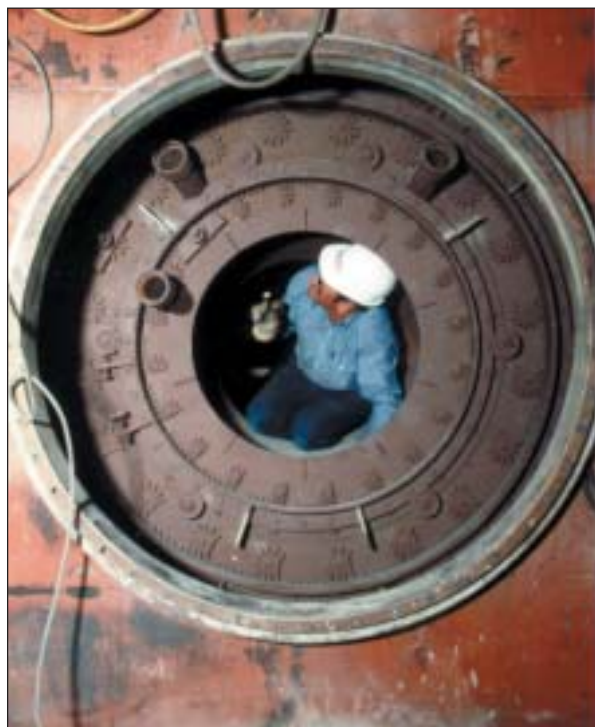
A worker inspects the support ring for the Foster Wheeler low-NO x burner installed in the boiler wall.
