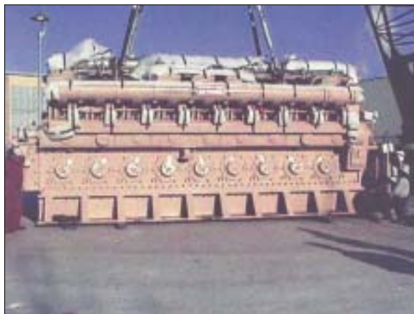
Shown is the Coltec coal-fired diesel being installed at the University of Alaska in Fairbanks.
