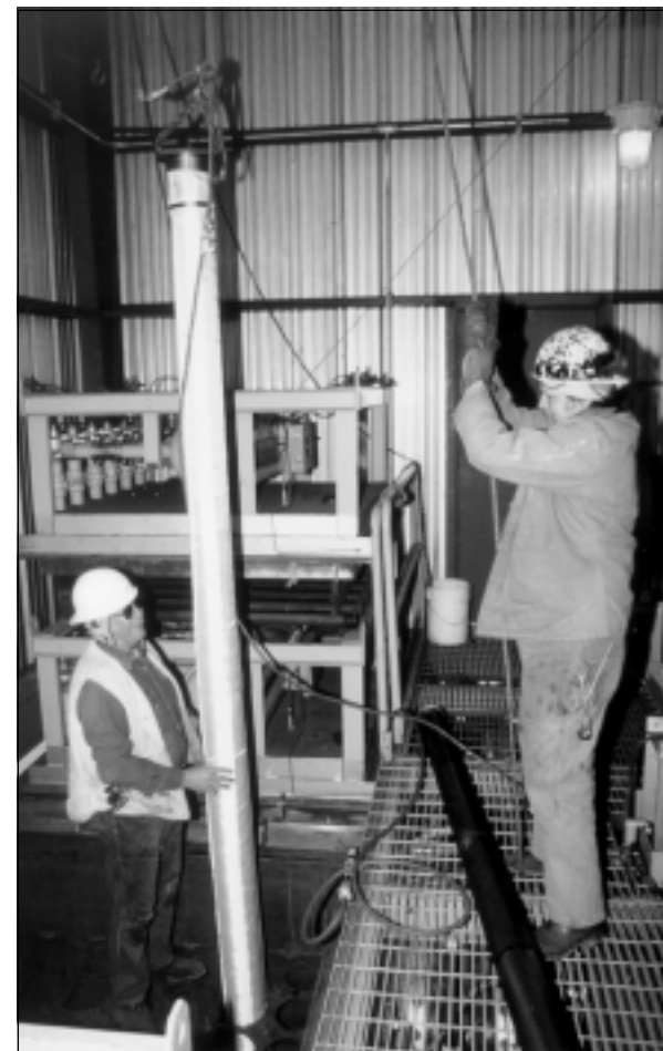
▲ Workers lower one of the catalyst holder tubes into a mounting plate in the penthouse of the high-temperature baghouse.
