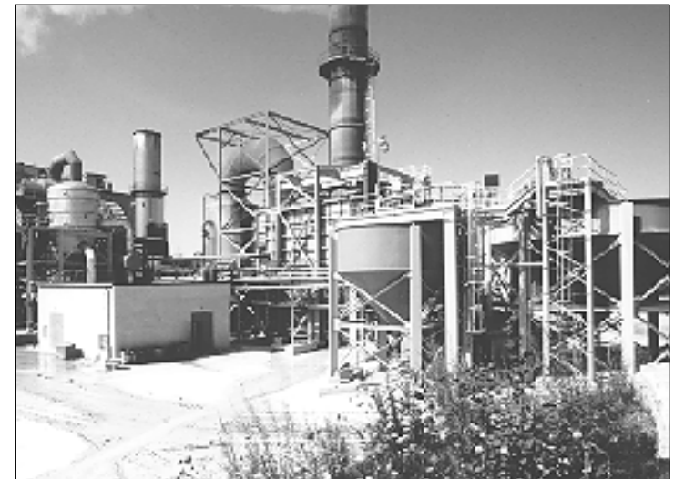
▲ The Passamaquoddy Technology Recovery Scrubber™ became a permanent part of the Dragon Products facility at the project's end.
