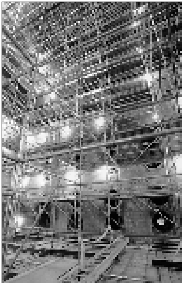
▲ Scaffolding and cell-burner penetration into the boiler wall are viewed from inside of a boiler.
