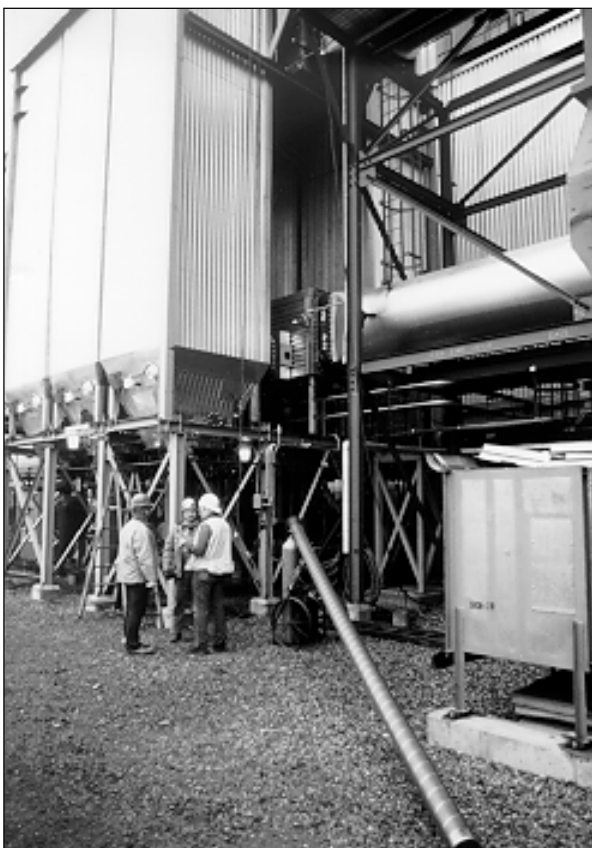
▲ The demonstration baghouse is installed on the back side of the power plant. Workers stand by the catalyst holder tube prior to lifting it into the penthouse.
