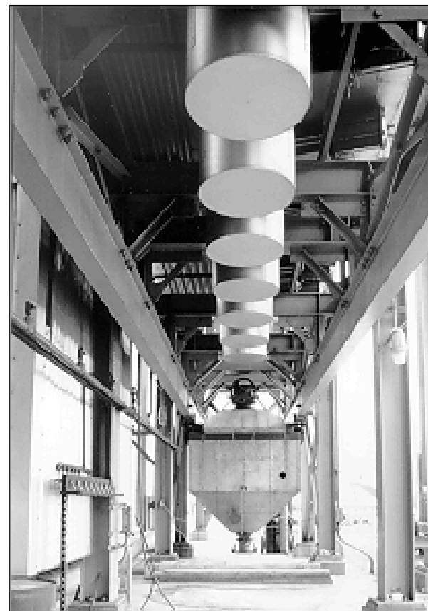
▲ The bottom portion of the SO 2 converter catalyst, with the catalyst dust collector hopper mounted on steel rails (center), is shown.
