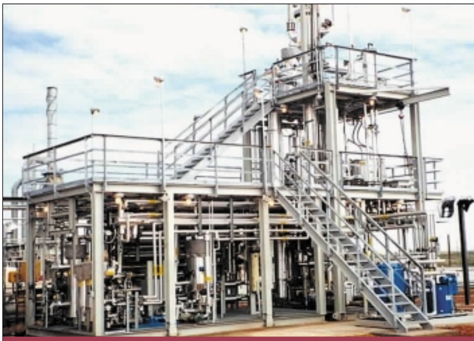
Figure 2: CrystaSulf® Pilot Unit Installed at West Texas Site
