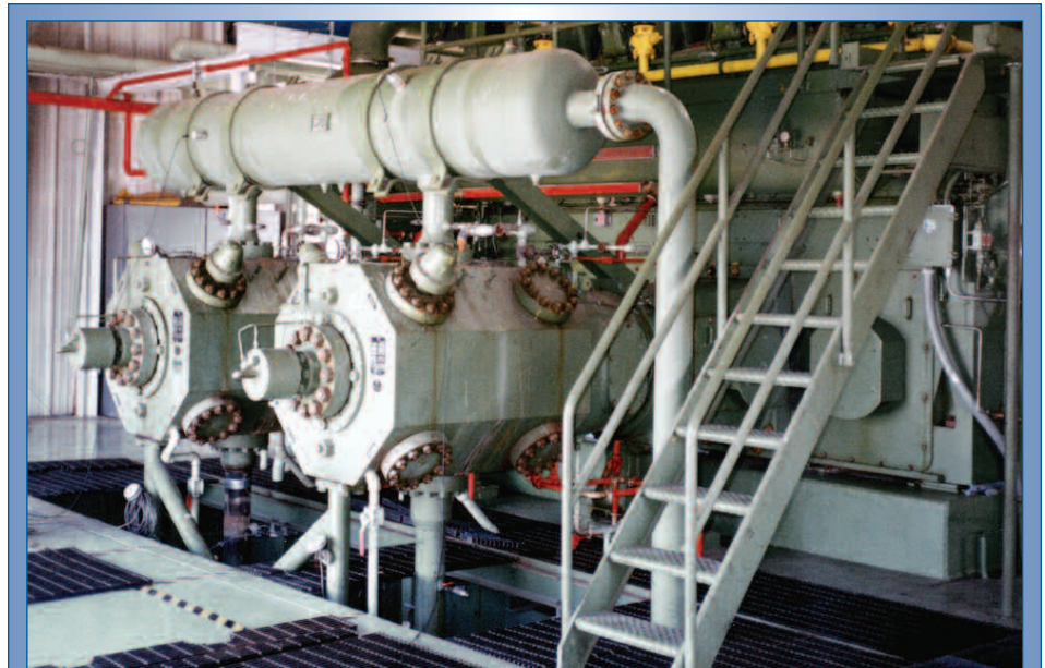
Figure 1. This slow-speed integral compressor is typical of the class of equipment that accounts for the majority of the U.S. pipeline infrastructure.
