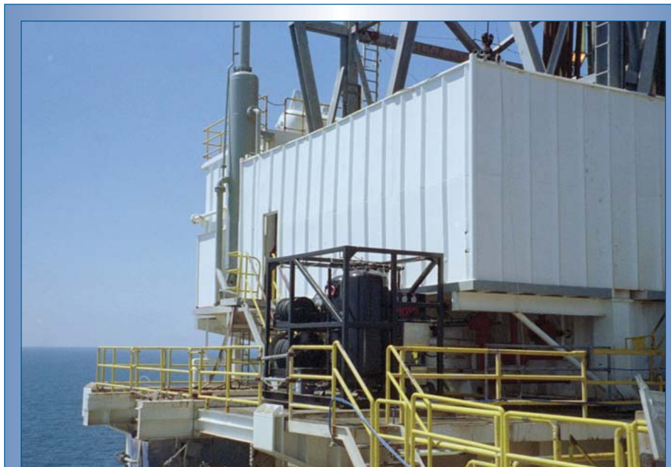
Figure 2. The cement pulsation unit (center) consists of the black, skid-mounted equipment.
