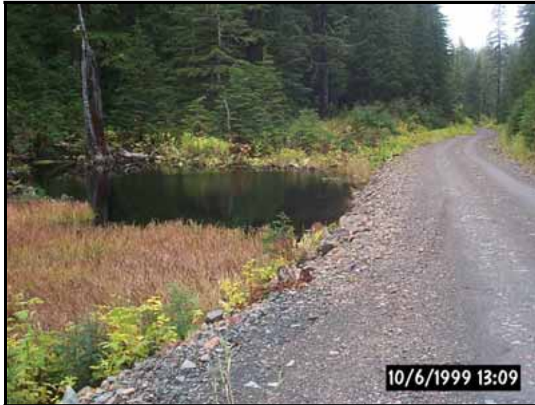
Beaver activity affecting road drainage.
