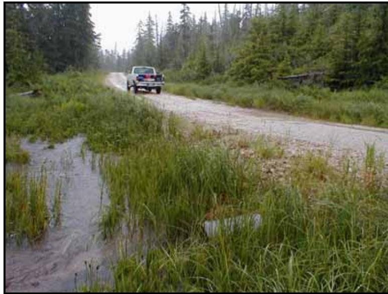
Location where a larger culvert is needed
