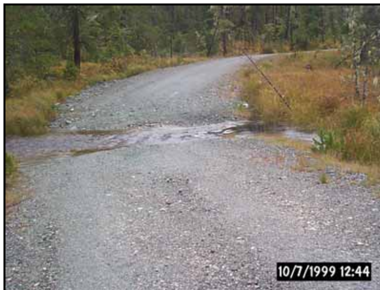
Running Water on Road Surface
