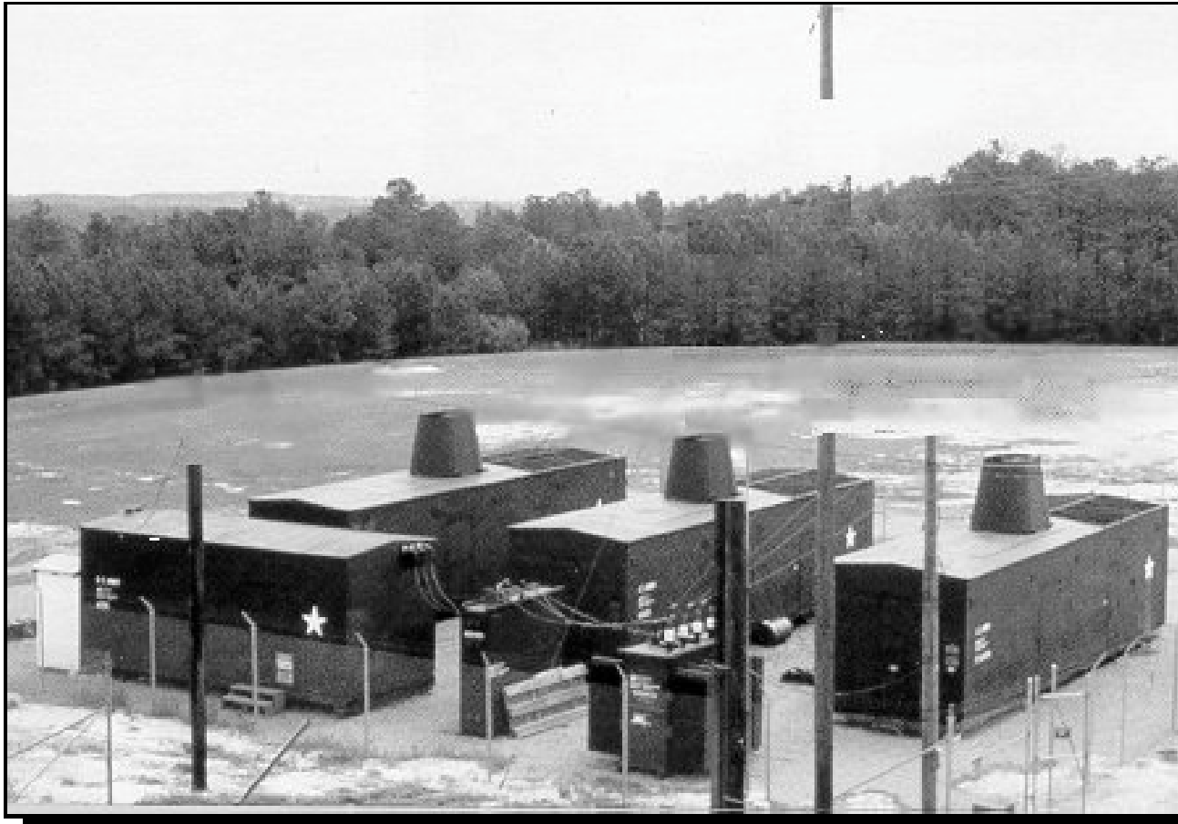
U.S. Army's Prime Power 4.5 MW Plant
