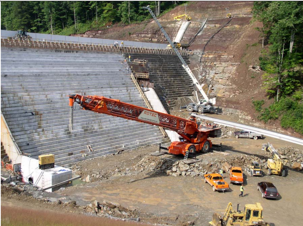
The Elkwater Fork Dam, in the Upper Tygarts Valley River Watershed, is a project to supply safe drinking water to 21,500 residents. This is a unique project to NRCS in West Virginia utilizing roller-compacted concrete (RCC) to provide the 54-acre water supply impoundment.
