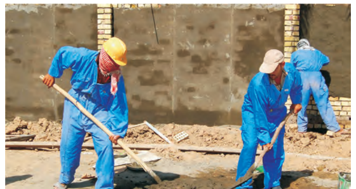
About 50 local Iraqis are on the construction crew building a 200 cubic meter per hour water compact unit and distribution network in Babil province.
