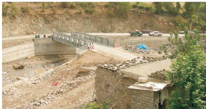
Rosti Valley Phase I bridge: During Phase I of the Rosti Valley project, a bridge was replaced that was critical for passage to 17 villages up and down the mountain river. This project also included the massive cleanup of debris from a flash flood in the spring of 2007.
