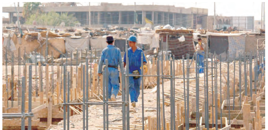
Construction is under way to build a $2.7 million fish market and a $2.4 million meat market in al Kut, Wasit Province.
