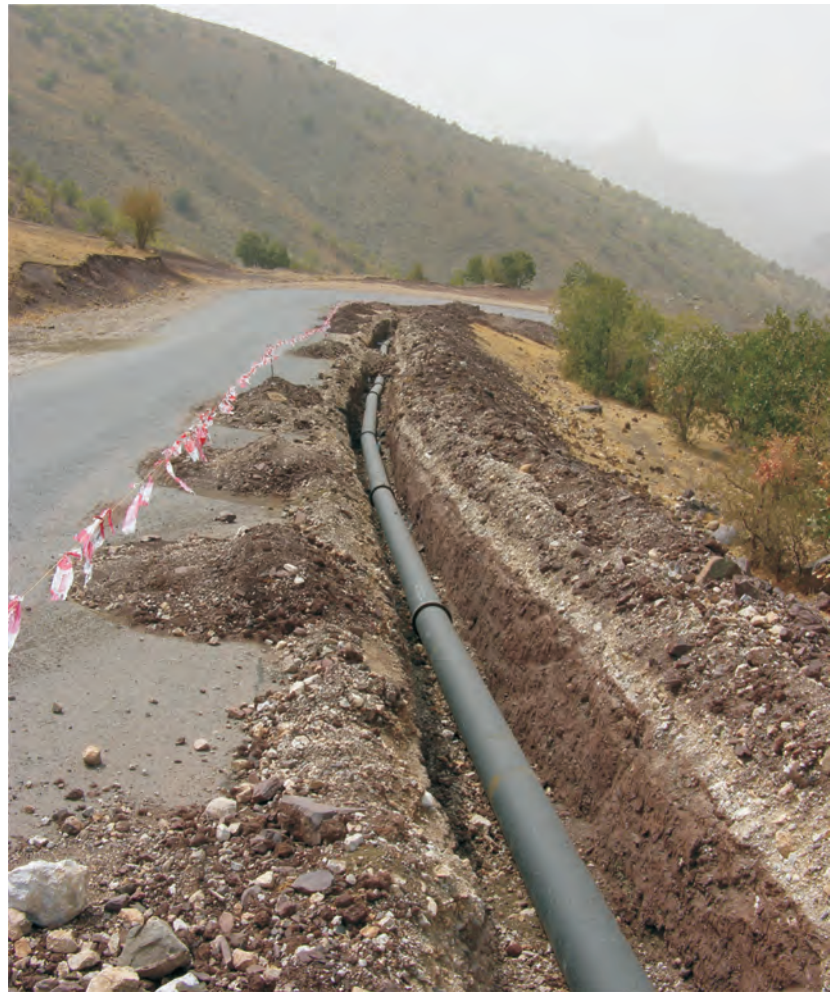
Five miles of pipe delivers mountaintop spring water to the town of Choman below and its two neighboring villages, where it connects to an existing water network.
