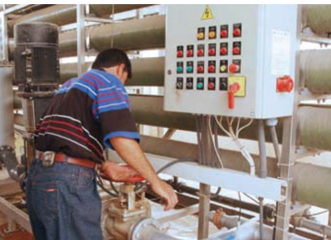
The plant operator runs the Reverse Osmosis unit now providing potable water to al-Zierji.
