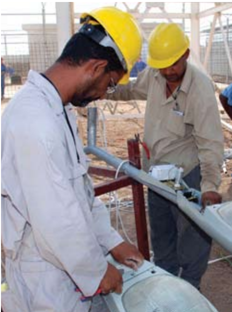
Above: Workers prepare security lights for the Modular Detainee Housing Unit area.
