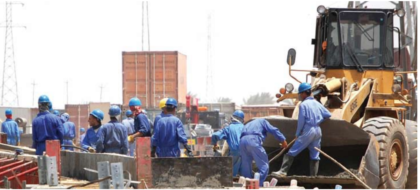
Workers place concrete during construction of a $25 million new 132 kV substation for the city of Diwaniyah.
