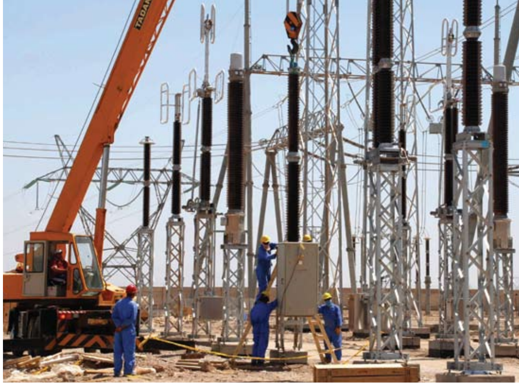
A 50-ton crane holds a 400kV insulator overhead as workers connect it to the bushing in the Qudas electrical generating plant switchyard
