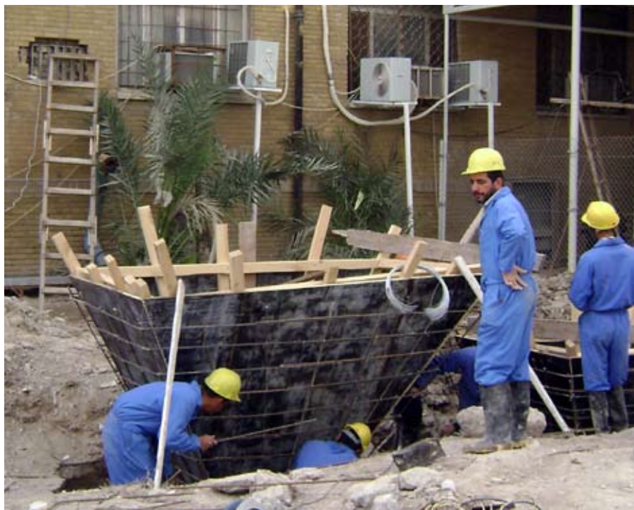
Iraqi workers install wooden forms and reinforcing bar for the construction of the two new manholes.
