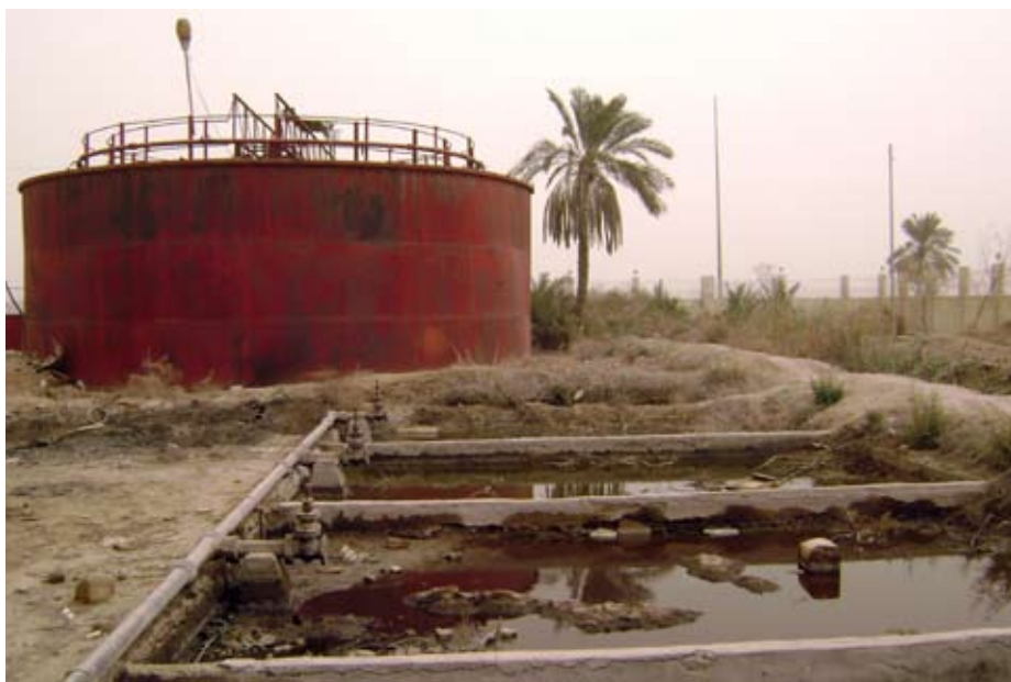
The old waste water treatment plant sits in disrepair, nonfunctional for more than 15 years.
