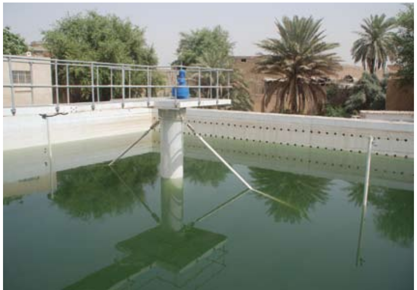
Potable water production is more than doubled from previous output at the Wahda facility in Baghdad.
