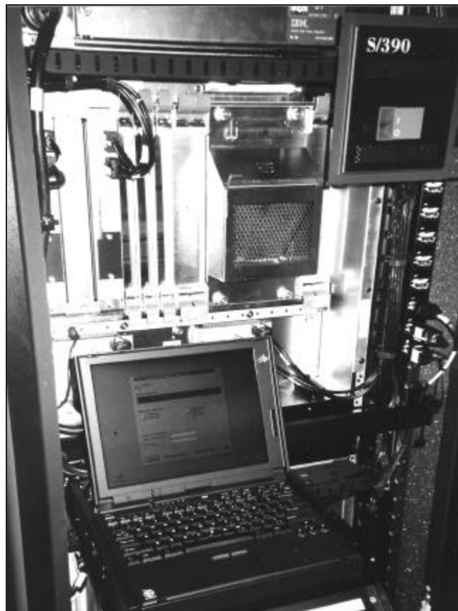
The HOCSR components include a laptop computer with windows-driven software to monitor and maintain the equipment.
