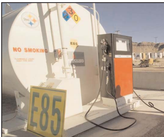
The Southwest view of the E-85 station and credit card reader.
