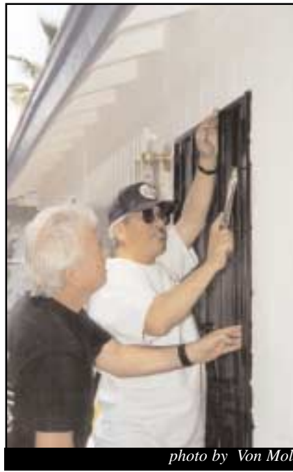
Team work is an important aspect of Christmas in April work. Dennis Finney (left) lends a helping hand as John Kitt installs a new security door on Marie Fields' home.
