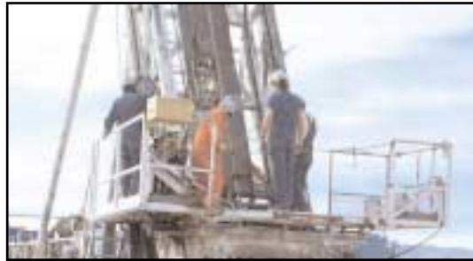
The crew removes tubing from a recently cemented borehole in preparation for demobilization.
