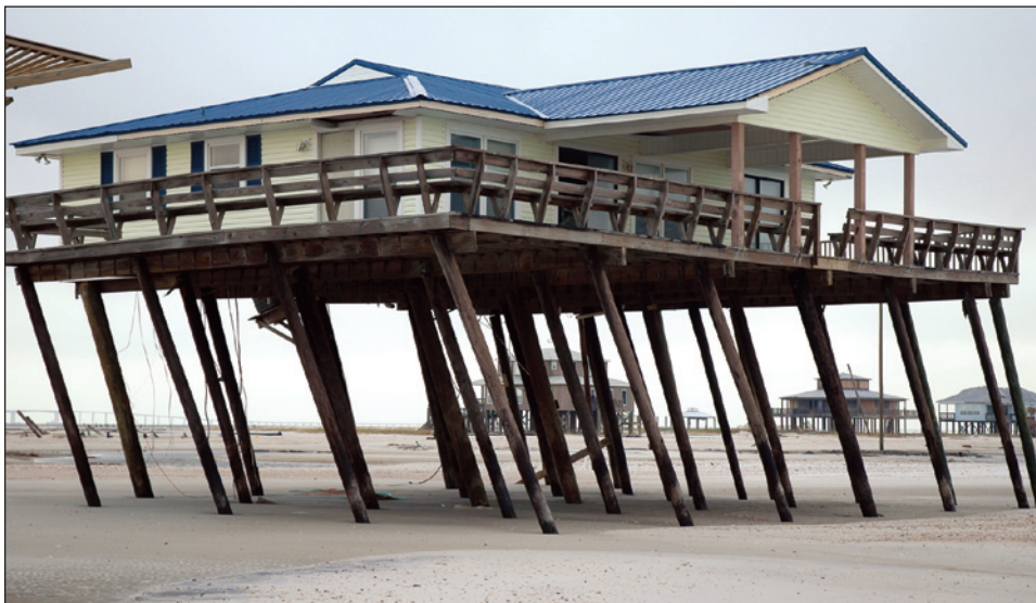
Figure 2-4. Near collapse due to insufficient pile embedment (Dauphin Island, Alabama)
