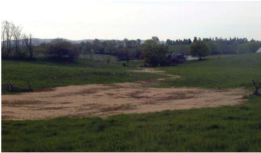
Figure 2. The restoration removed an intermittent pond and berm, improving drainage in the areas where cattle congregated. To disperse cattle, managers routed runoff to two troughs. The area was re-graded and seeded to complete the project, safeguarding groundwater and streams of the Chesapeake Bay watershed. NPS
