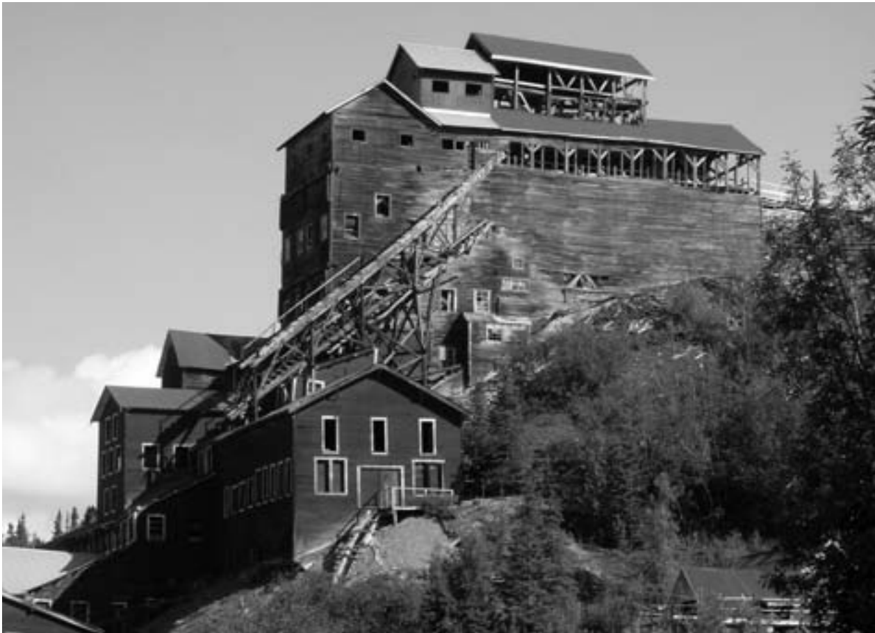
Figure 4. The mill building stands prominently on the hillside in Kennecott. The National Park Service has deemed this building a high priority for stabilization. COPYRIGHT STEVE TAYLOR
