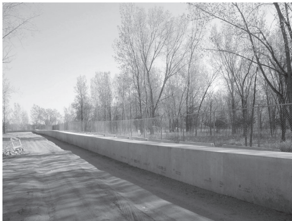
Figure 3: Example of a Vehicle Barrier System
