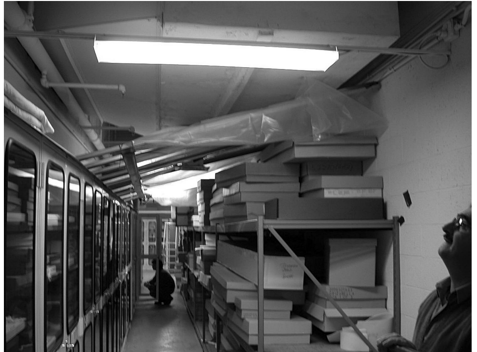
Figure 15: Leak in the Room 4303 (History Storage Room) at the National Museum of American History
