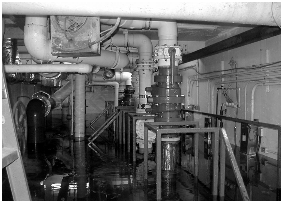
Figure 8: Flooded Mechanical Room at the National Zoo
