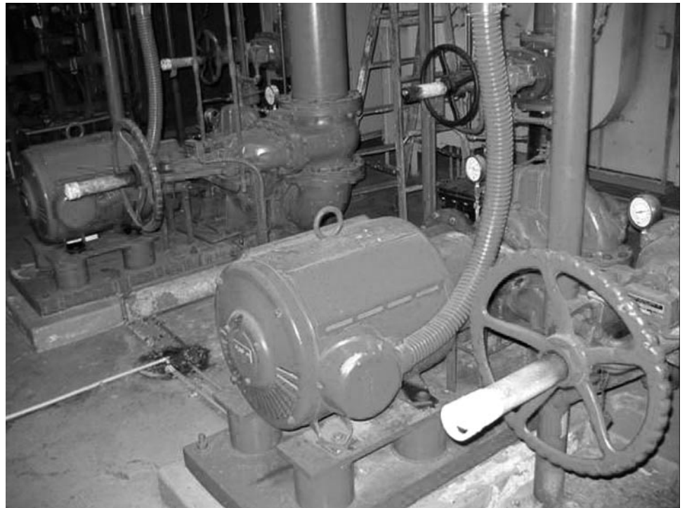
Figure 13: Antiquated Fire Suppression System, National Air and Space Museum
