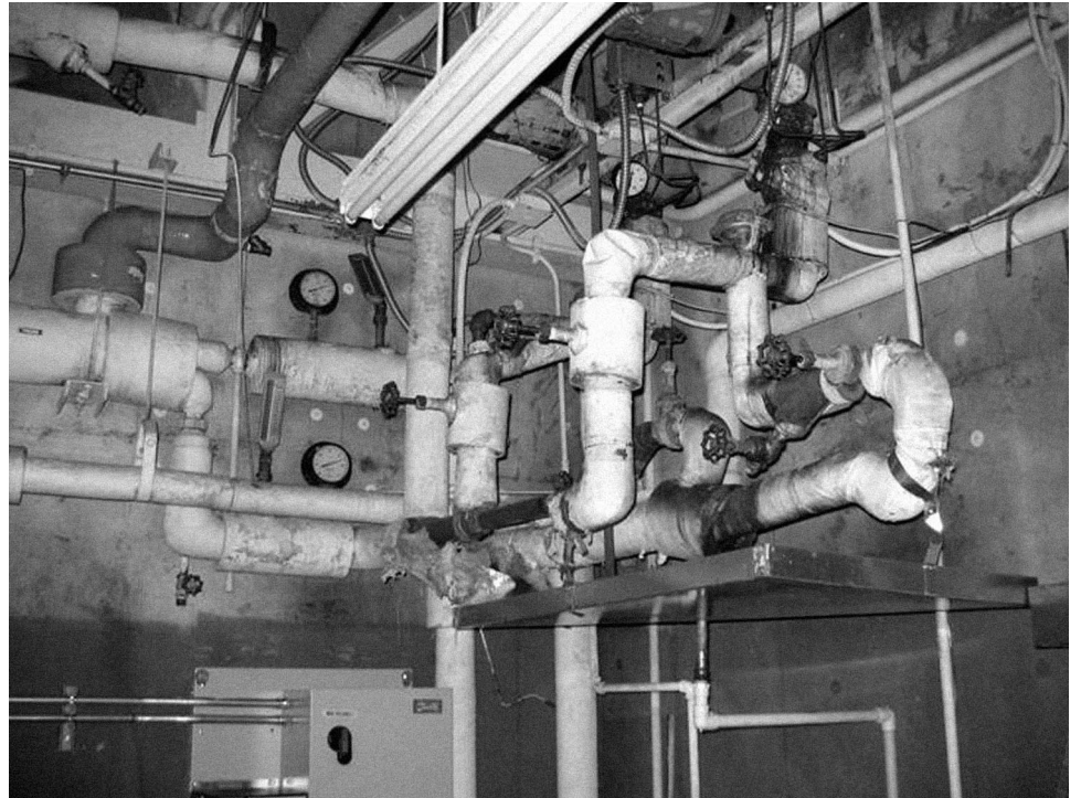
Figure 12: Failing Heating, Ventilation and Air Conditioning System at National Air and Space Museum
