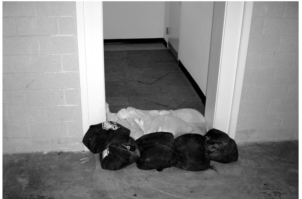
Figure 14: Flooding in High-Voltage Room, National Museum of American History
