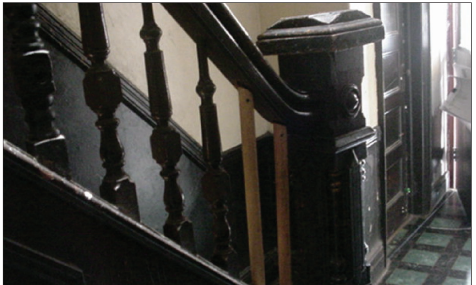
Figure 17: Property 2—“$1,082 Wooden Dowels”
