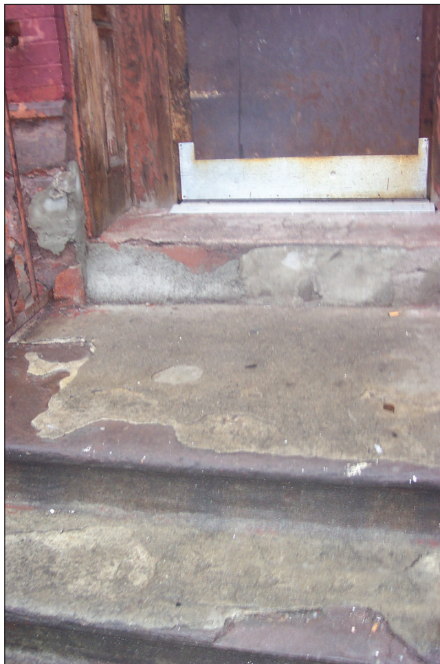
Figure 22: Property 4—$3,978 in Stoop “Repairs”
