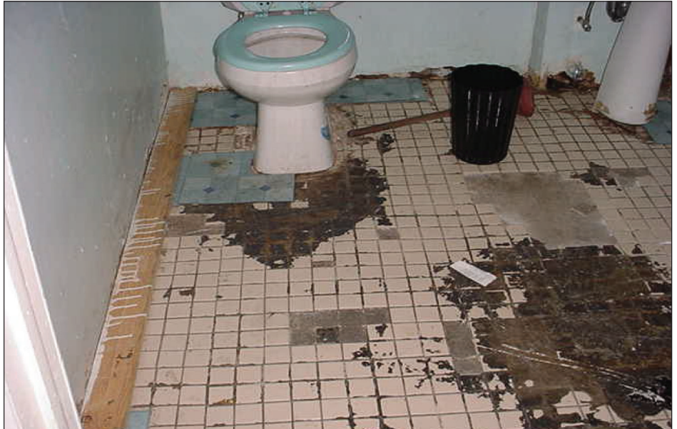
Figure 12: Property 1–“New” Bathroom Floor
