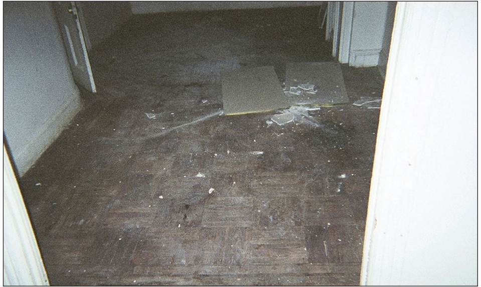
Figure 19: Property 3—"New" Dining Room Ceiling on Floor
