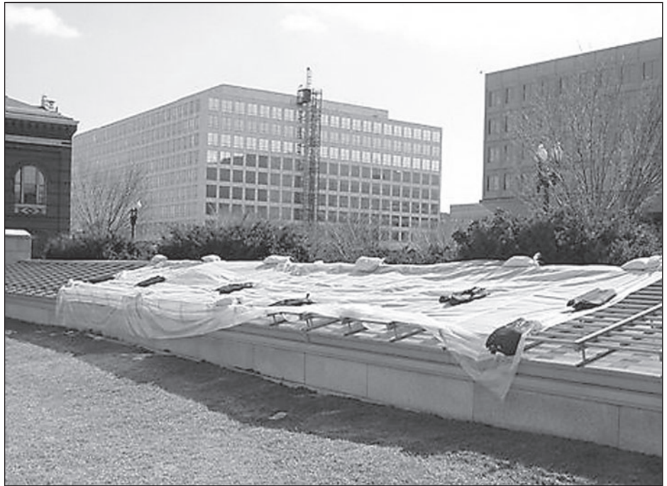
Figure 11: Leaking Skylight over the Museum of African Art
