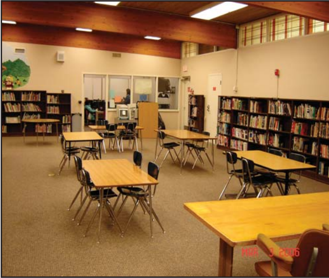
AFTER: The library at Sunset Elementary School after the new lighting was installed is brighter and and evenly distributed. The schools expects to save 47 percent of its energy use.
