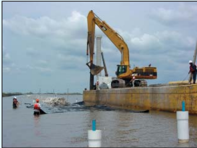
Placement of the bottom layer of geotextile fabric over existing foundation in native foundation displacement reach. (USACE)
