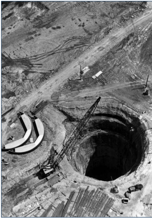
Construction of the B-2 site required the excavation of a 180-foot-deep hole, pictured here in 1965. (Source: Glenn Research Center, file photo number 01264)
