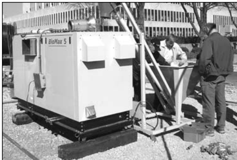
The BioMax generator gasifies wood pellets to produce electricity cleanly.
