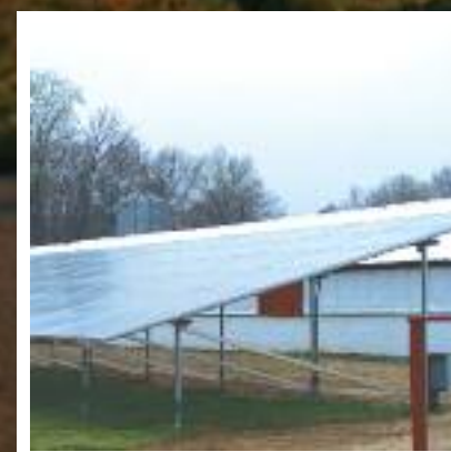
Laurel - University of Delaware Solar Panel Poultry House.
