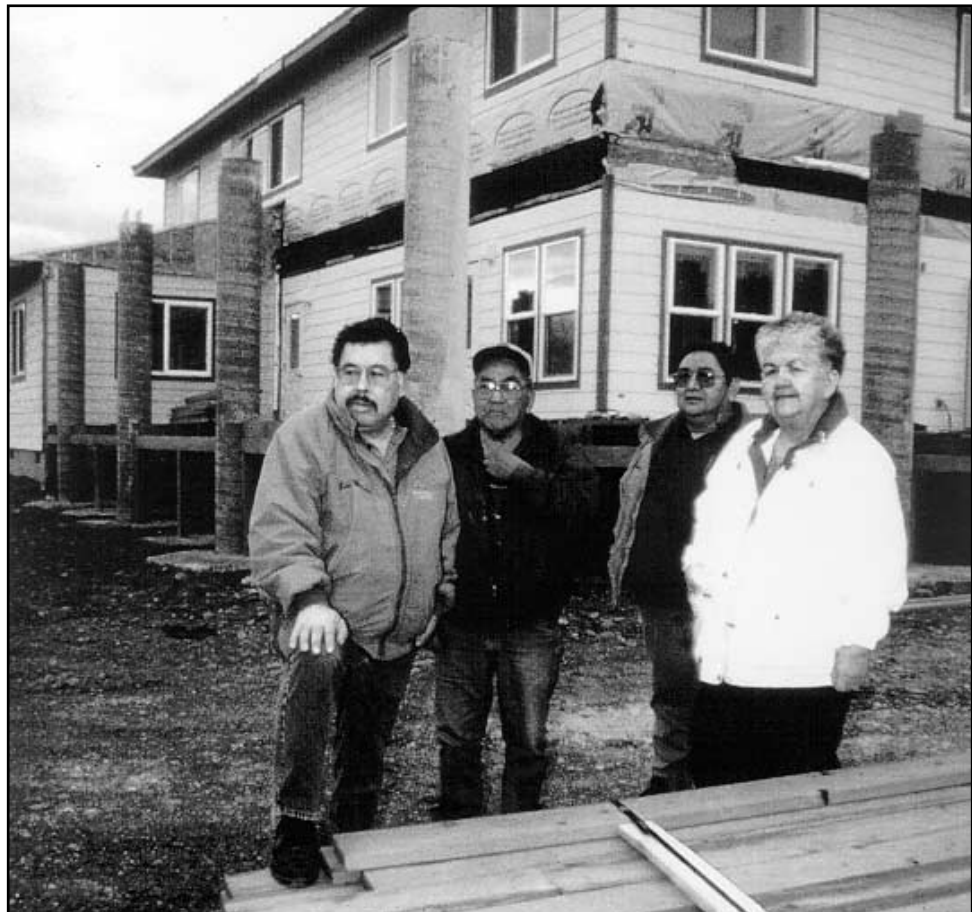
Quileute Tribe members on the construction site of their new Natural Resources building. When the old building was condemned, a local bank agreed to make them a loan. However, because the building would be on Tribal Trust land, the lender required a guarantee from RHS to properly secure the loan. The Community Facilities Program guaranteed a loan for $385,000 in September 1999, and the building was completed in the spring of 2000.
