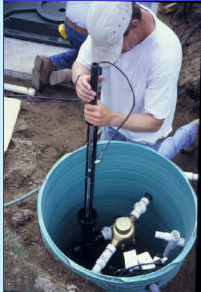
UV light disinfection unit
