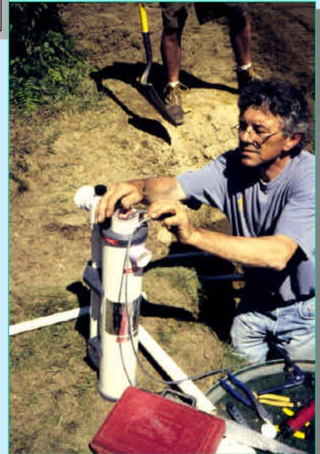
Ultraviolet (UV) light disinfection unit
