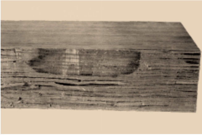
Figure 9.2—Dirt and stain inside a check, a certain indicator that the check was open during air drying.
