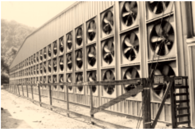
Figure 5.4—Typical fan shed used in a mill in Appalachia. Drying must be carefully monitored to prevent checking.
