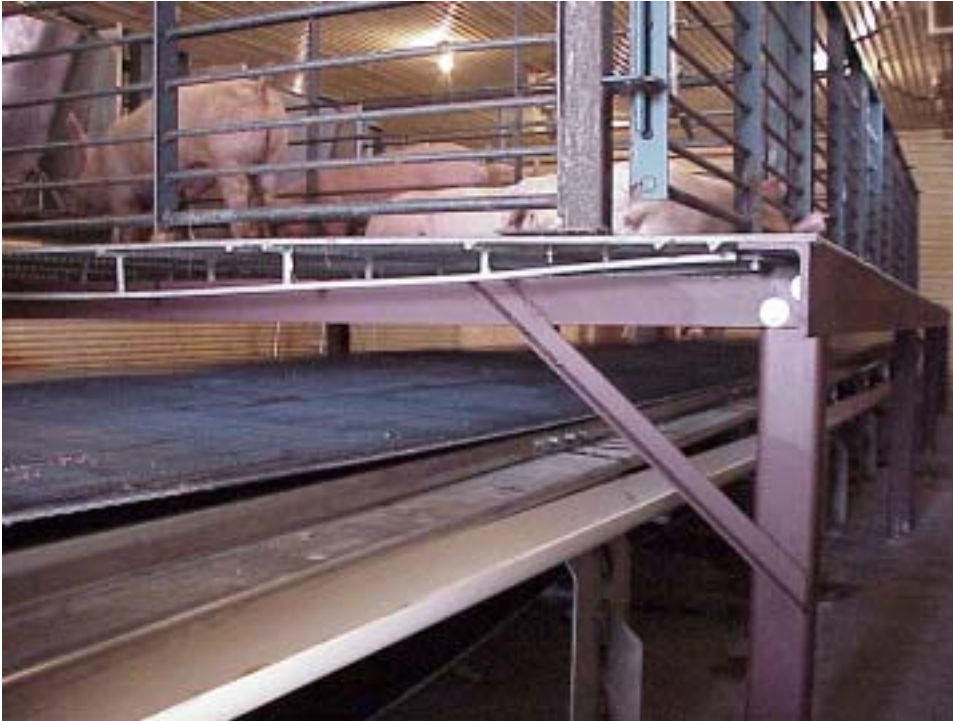
Figure 2. Belt system after solids removal.
