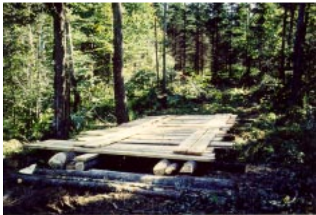
Figure 5.—Abutment logs below a log stringer bridge (approach yet to be constructed).
