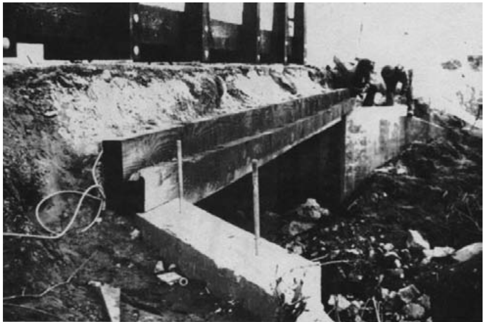
Figure 15-21. - Anchor bolts are placed in the concrete wingwalls that match predrilled holes in the timber deck panels.
