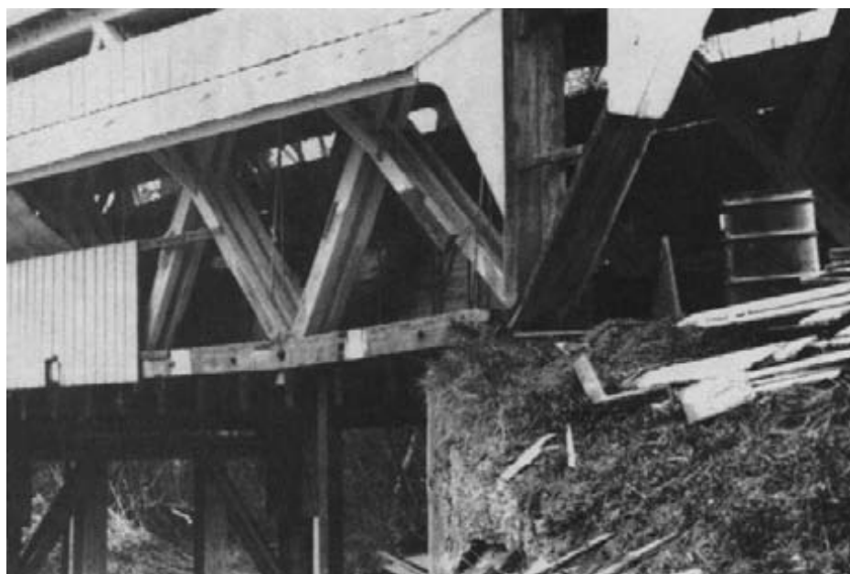
Figure 15-33. - Broken lower chords at two of the four corners prompted the replacement of some existing truss members.
