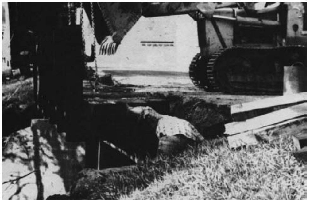
Figure 15-23. - A prefabricated deck panel is lifted onto the abutments. Each panel was prefabricated to fit each bridge.
