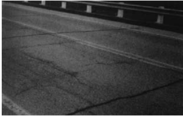
Figure 15-38. - Breakup of asphalt pavement because of delamination of the nail-laminated timber deck.
