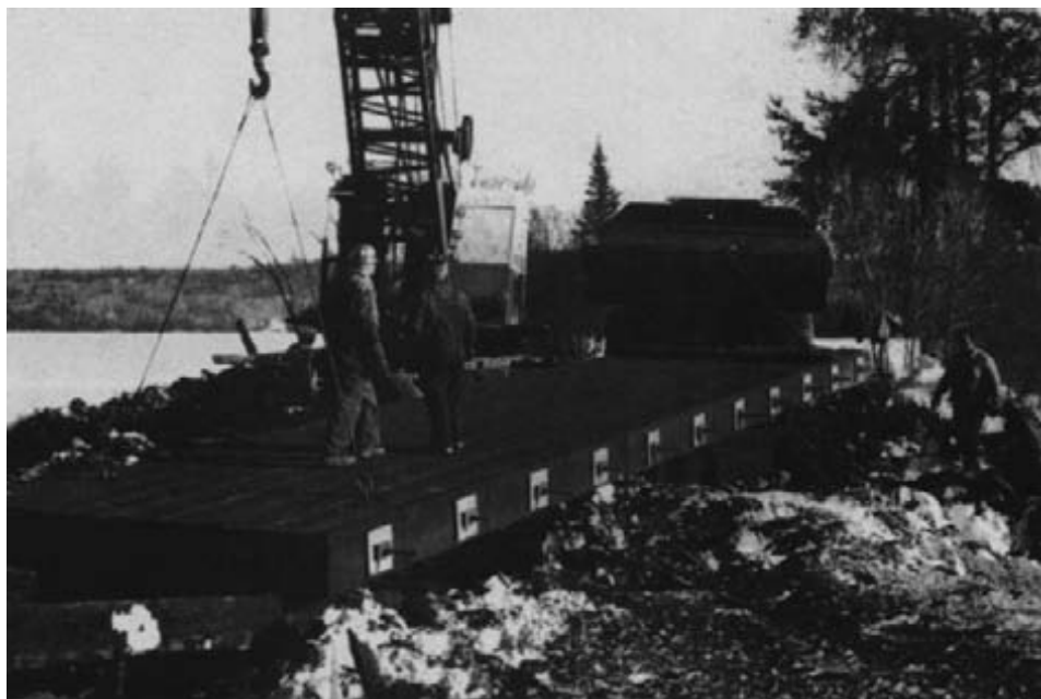
Figure 15-79. - One of the prefabricated, prestressed, bridge deck panels is lifted into position on the treated-timber crib abutments.
