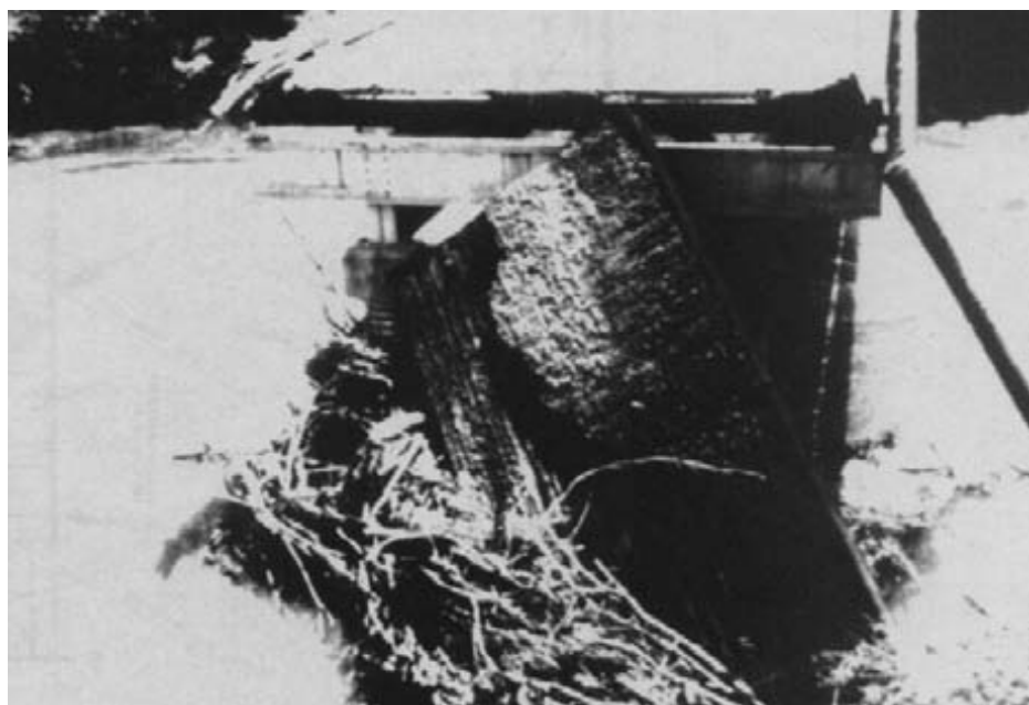
Figure 15-57. - Close-up of the collapsed longitudinal nail-laminated lumber approach span.
