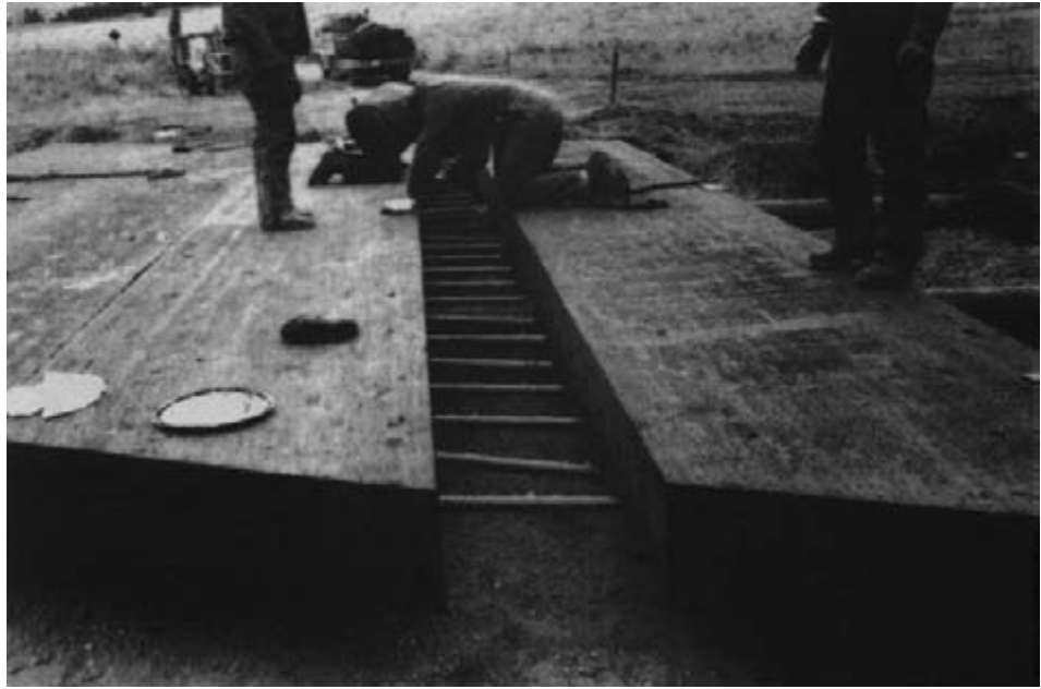
Figure 15-71. - Steel dowels are aligned before joining the fourth panel. The dowels are 1-1/2 inches in diameter, 19-1/2 inches long, and are spaced 12 inches on center.
