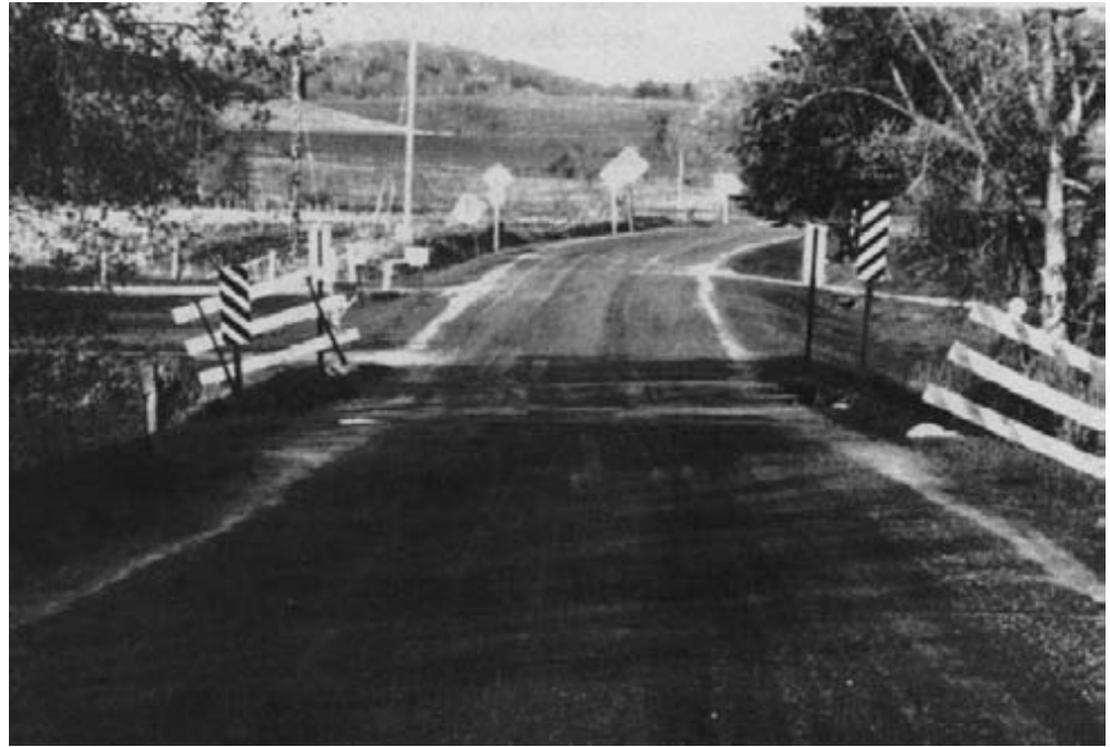
Figure 15-18. - Typical concrete bridge on Pepin County Trunk Highway Z before rehabilitation. The bridges were adequate hydraulically and structurally, but did not meet minimum standards for roadway width.
