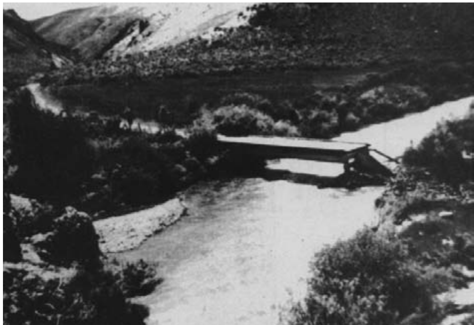
Figure 15-56. - Collapsed span and breached approaches of the existing bridge.
