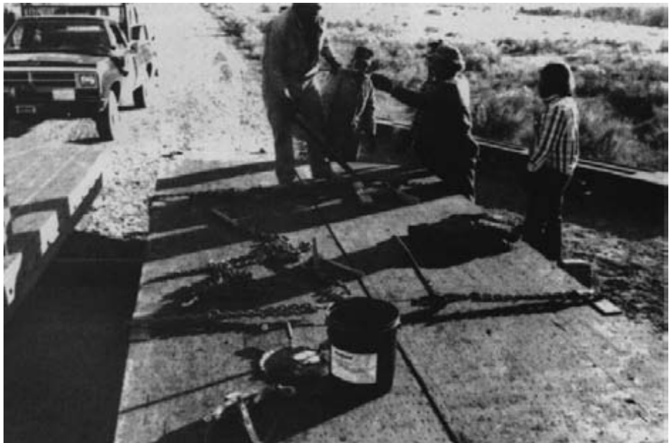
Figure 15-70. - Another view of the first two panels being pulled together. Note the corner protectors under the come-a-long chains and the can of roofing cement on the deck. All panel joints were sealed with the roofing cement before being pulled together.
