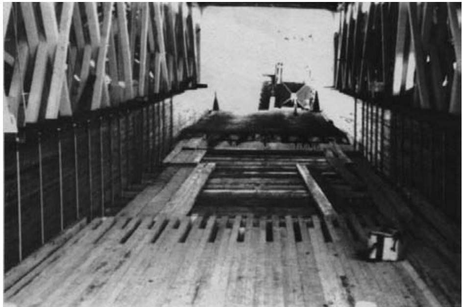
Figure 15-35. - A view inside the bridge showing the glulam girders, floorbeams, and longitudinal nail-laminated lumber floor. The existing floor, still in place at the far end of the roadway, was removed in sections to facilitate construction.
