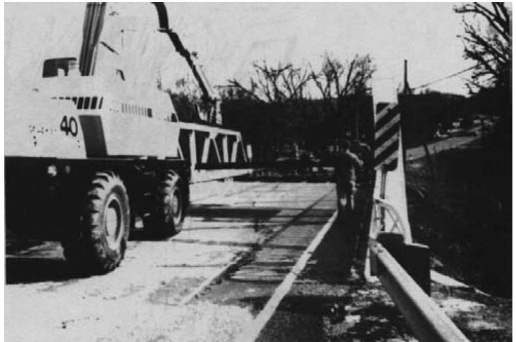
Figure 15-50. - New, prefabricated treated-timber deck panels were placed with a hydraulic excavator. The panels were designed to fit transversely on the stringers and were placed without removing the existing railing.
