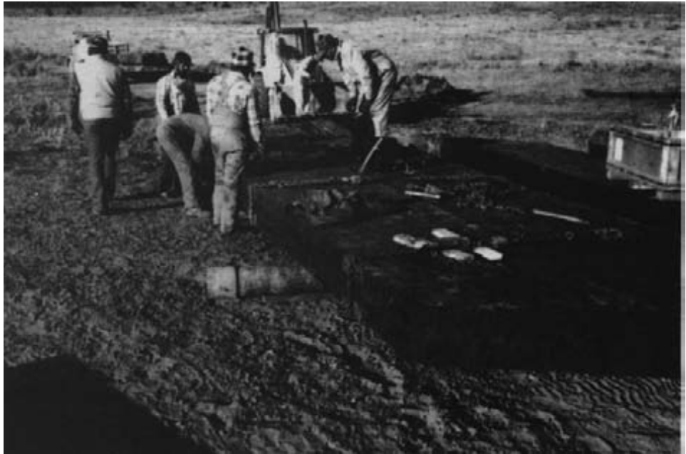
Figure 15-69. - The first two panels of the new bridge are interconnected with steel dowels and pulled together with a come-a-long. Because the crossing was skewed, the doweled panels could not be assembled on the abutments. Assembly was completed adjacent to the site on two well casings to facilitate assembly and lifting.
