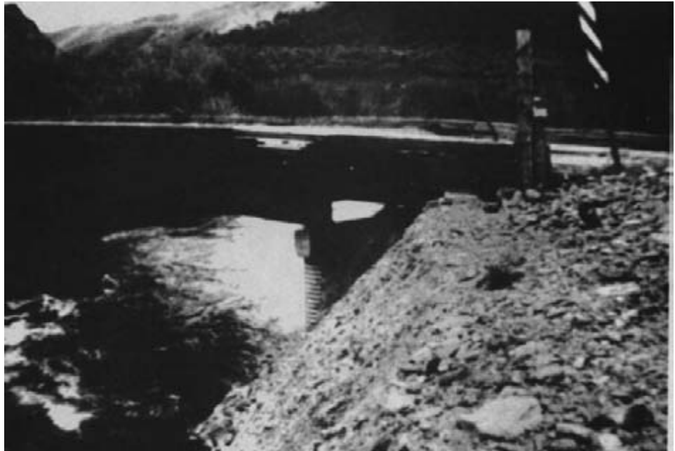
Figure 15-58. - The temporary repair made to the bridge consisted of replacing the approach embankment and lifting the nail-laminated approach span back into position.
