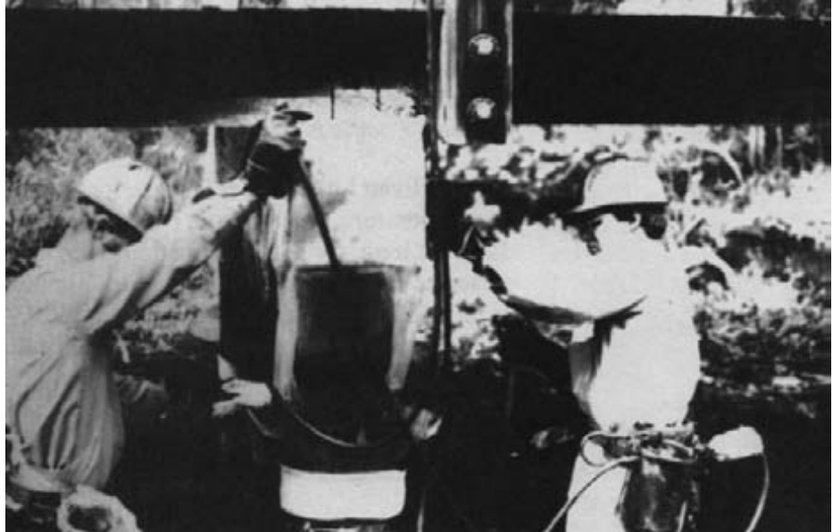
Figure 15-12. - Two-person crew injects liquid wood preservative solution into piles and caps. Note the safety backflow valve on the worker's belt.
