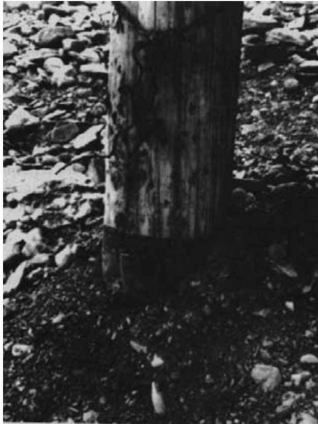
Figure 15-16. - Timber pile after treatment of the soil contact area. The treated portion of the pile was wrapped in waterproof paper to prevent potential soil contamination.
