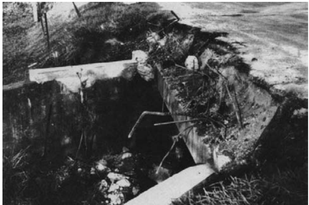
Figure 15-19. - The first step in the rehabilitation was removal of the concrete curb and railing. Next, a concrete seat was poured on the wing walls to support the additional deck width. This bridge also had 2 feet of overburden removed as part of the contract.
