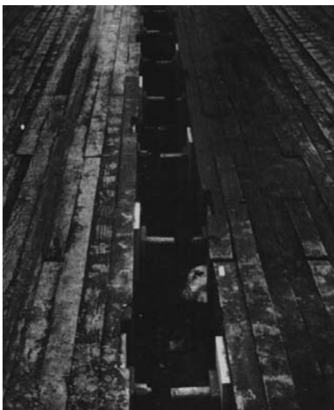
Figure 15-80. - Prestressing rods protruding from the two prefabricated deck panels before connection. The rod opposite each coupler was released and threaded into the coupler. After all couplings were made, the released rods were restressed, causing the deck panels to be stress-laminated together as an integral bridge deck.
