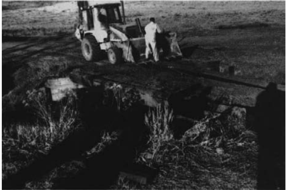
Figure 15-67. - The existing deck was carefully removed in sections to avoid damage to the treated-timber abutment caps.
