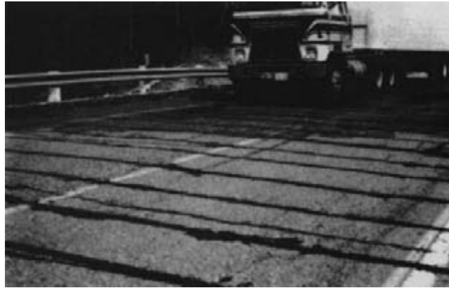
Figure 15-42. - Top prestressing bars installed in grooves cut in the asphalt wearing surface of the North Pagwachuan River Bridge near Terrace Bay, Ontario.
