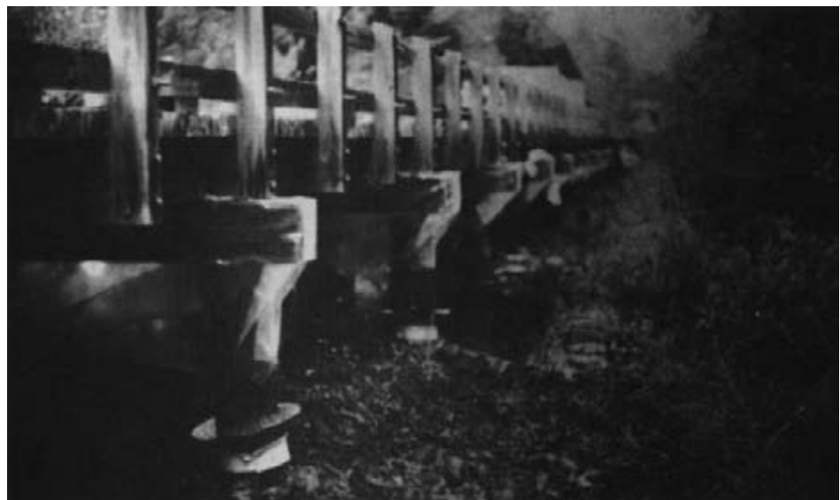
Figure 15-11. - Bridge draping for spillage protection, in place and ready for preservative injection.
