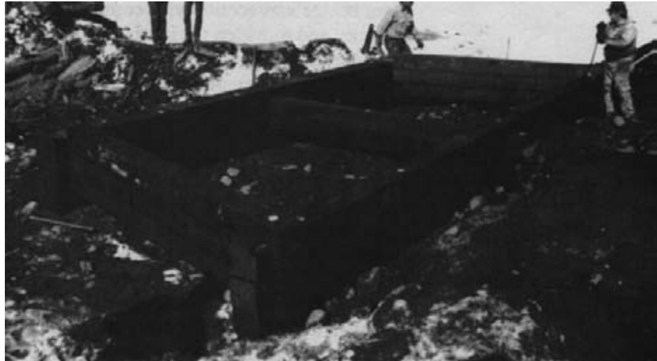
Figure 15-78.-The new crib abutment under construction using precut and creosote-treated Douglas-fir timbers. The only field fabrication involved drilling holes in the timbers for drive spikes used for connections. Such penetration of the protective envelope should have been avoided by drilling before pressure treatment (photo courtesy of Wheeler Consolidated, Inc.).
