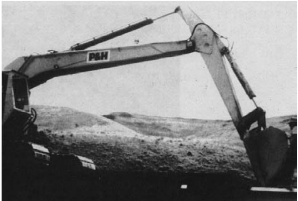
Figure 15-64. - Backhoe pushes panels together after dowels have been aligned. A large timber block was placed across the panel edge to prevent damage from the backhoe bucket.
