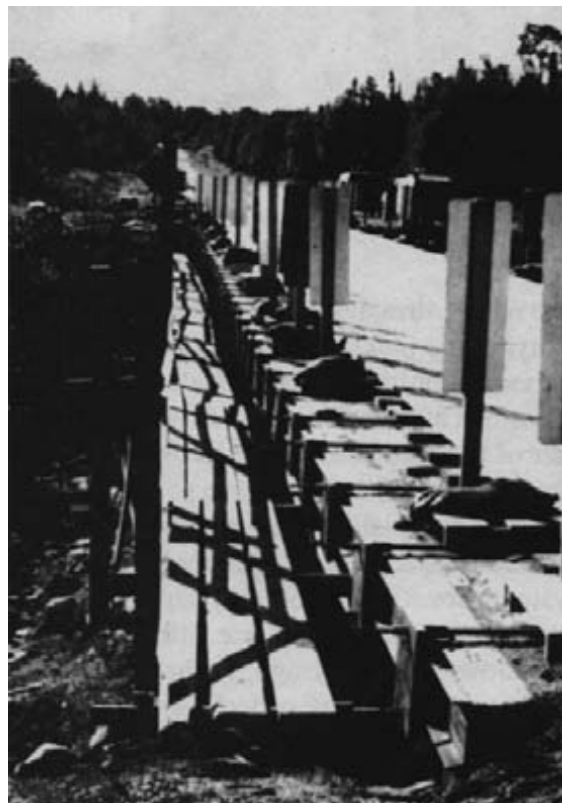
Figure 15-43. - Temporary plank surface placed over prestressing bars during construction at the Pickerel River Bridge.
