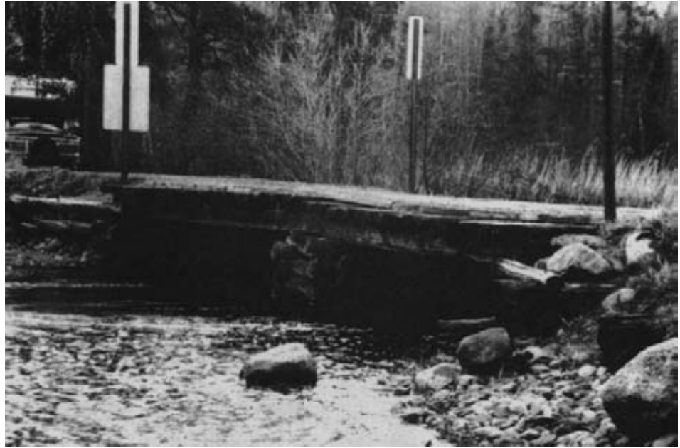
Figure 15-76. - The existing single-lane bridge was a simply supported, two-span, untreated-timber beam bridge supported by log cribbing (photo courtesy of Wheeler Consolidated, Inc.).
