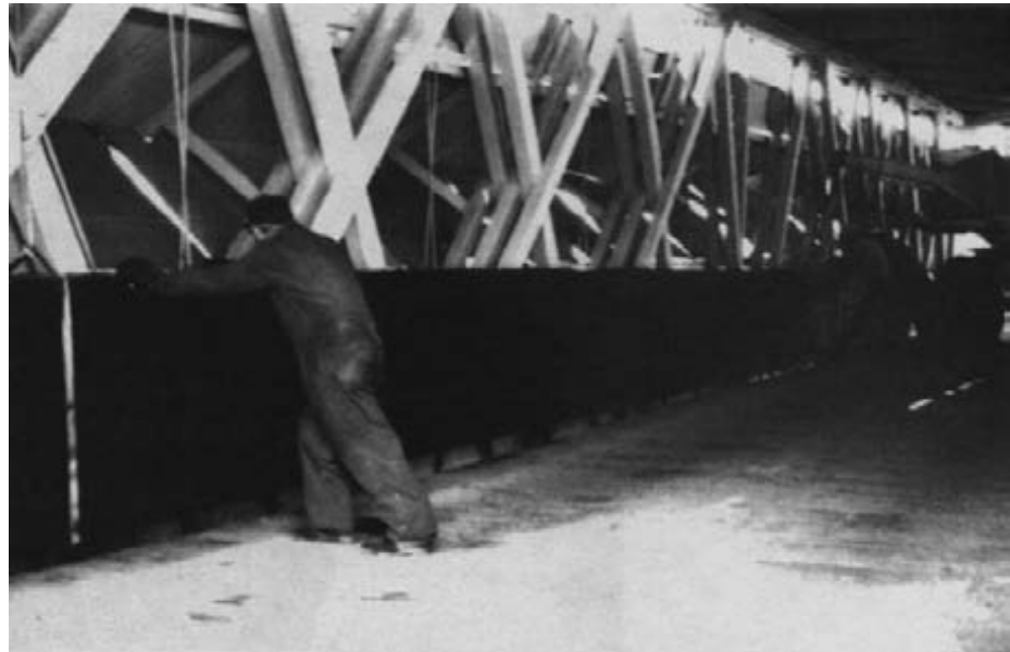
Figure 15-29. - Support for the roadway was obtained by installing two pressure-treated glulam girders inside the existing bridge, one along each side of the roadway.
