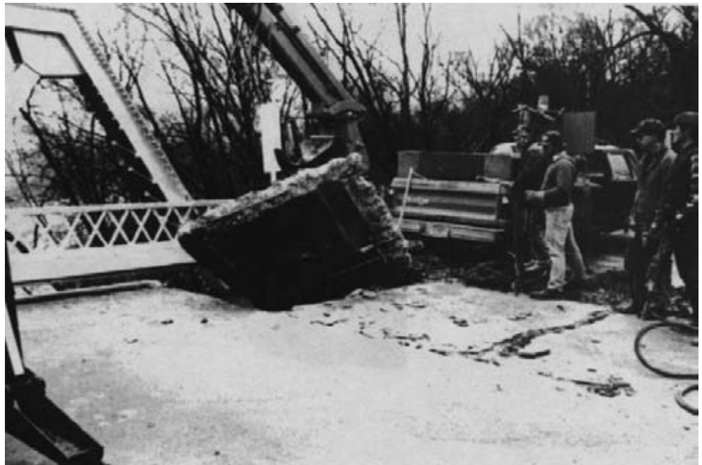
Figure 15-48. - The concrete deck was removed in approximately 5-foot-square sections by the Sauk County Highway maintenance crew. The concrete was broken using jackhammers, and reinforcing bars were flame cut. The sections were lifted and loaded on the trucks with a hydraulic excavator.
