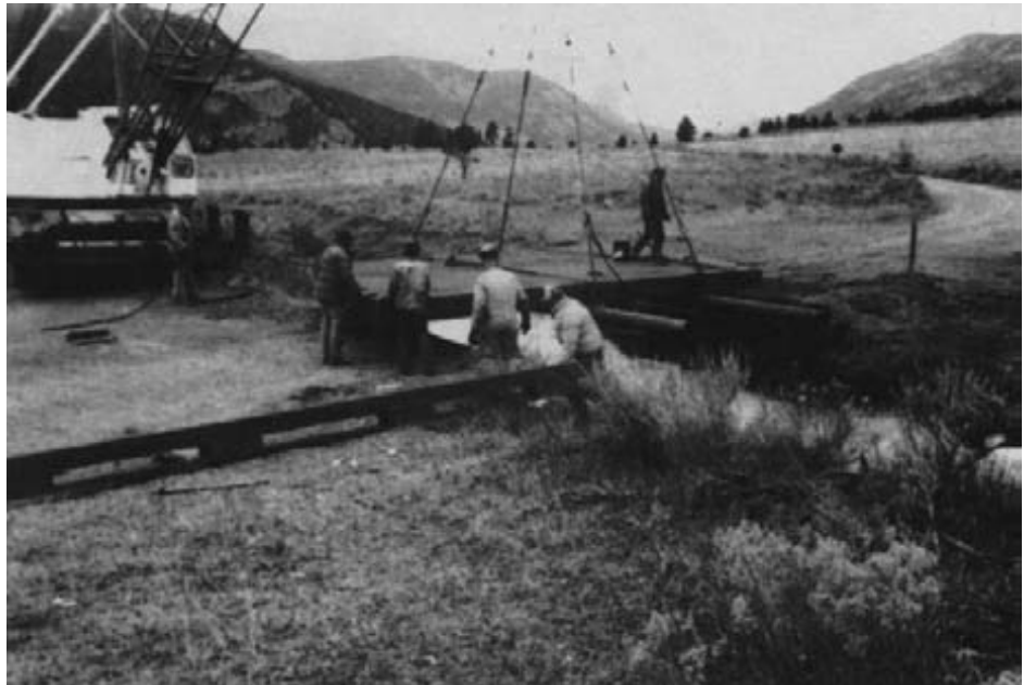
Figure 15-72. - The completed deck, resting on the well casings, is lifted into place on the abutments. Note that the curbs have been preassembled adjacent to site.
