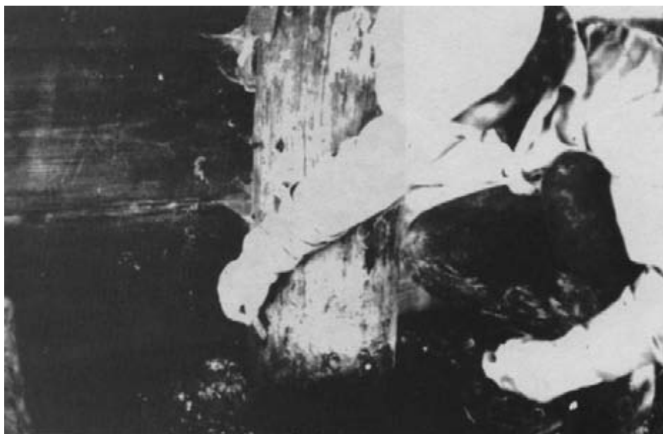
Figure 15-6 - Insertion of solid preservative cartridges into a timber pile. Note the use of rubber safety gloves.
