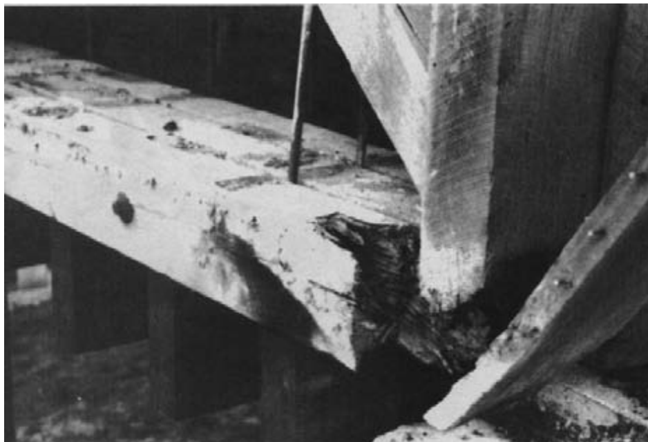
Figure 15-32. - Severe deterioration at each corner of the bridge was one cause of the poor truss alignment. New floorbeams were extended beyond the girders to help support each truss.
