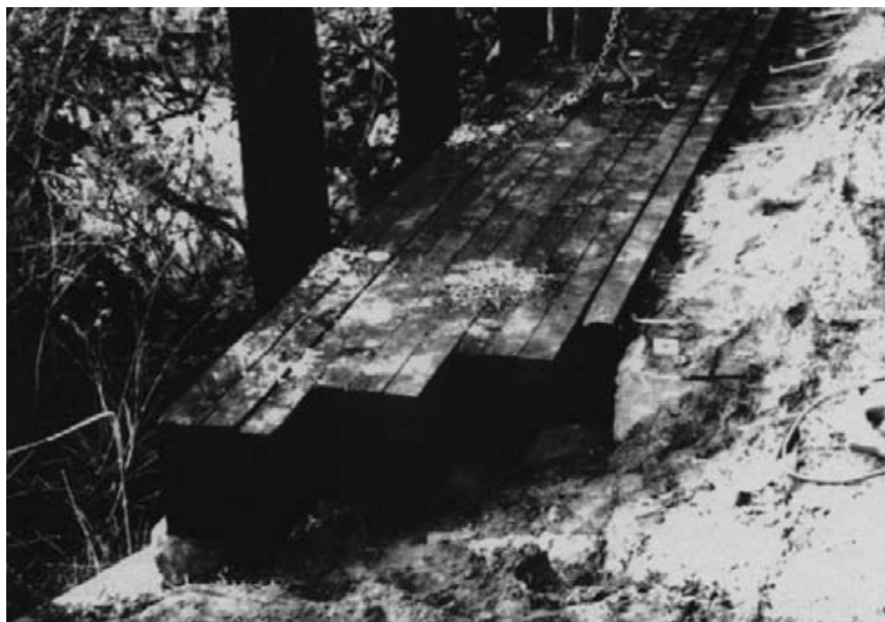
Figure 15-25. - A panel in final position. The ship-lap joint between the deck panel and first plank are interconnected with 5/8-inch-diameter by 13-inch-long drive spikes placed vertically through the joint.
