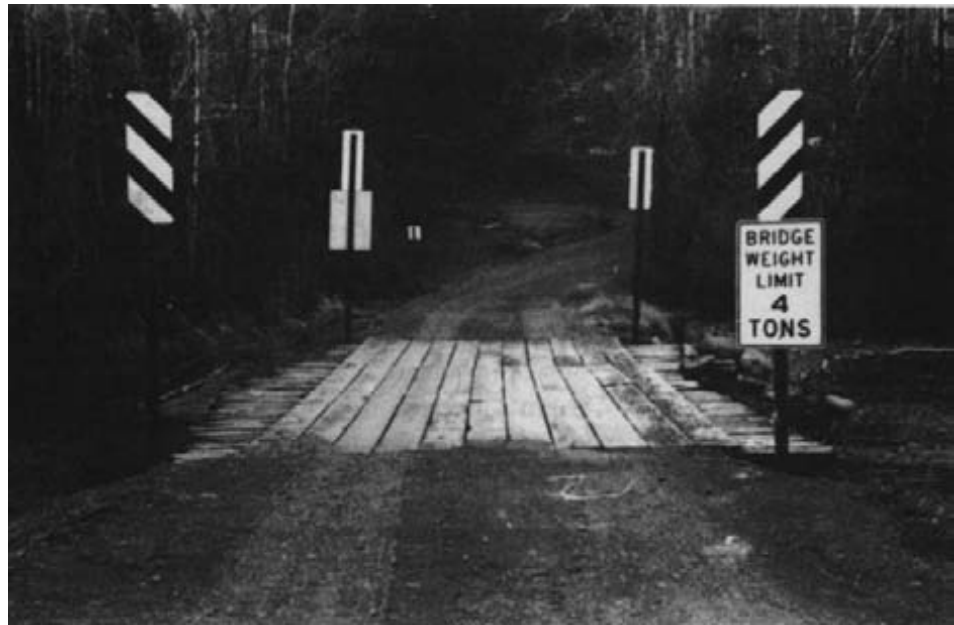
Figure 15-77. - The existing bridge was structurally deficient and load-posted. In addition, it was too narrow and lacked curbs and railing (photo courtesy of Wheeler Consolidated, Inc.).
