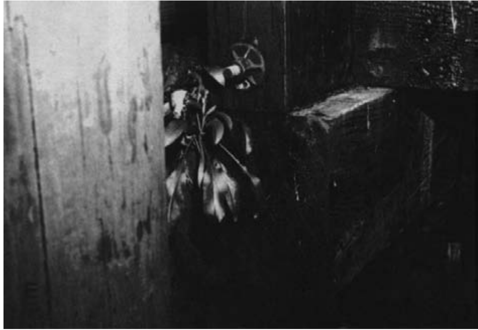
Figure 13-22. - Visual signs of potential deterioration (continued). (E) Plant growth.
