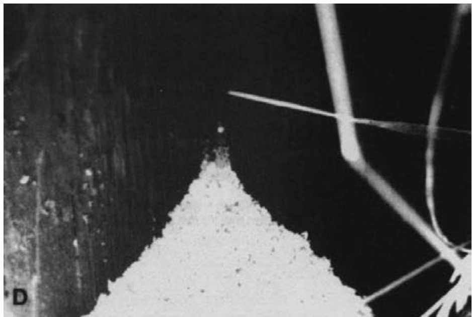
Figure 13-22. - Visual signs of potential deterioration (continued). (C) Water staining. (D) Insect activity (powder posting).
