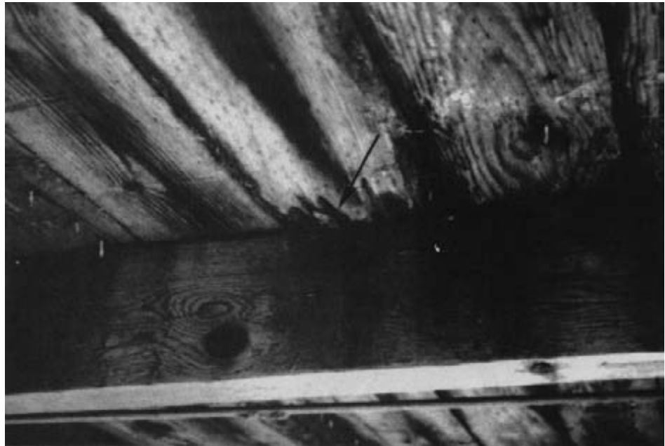
Figure 13-47. - Decay on the underside of a spike-attached lumber plank deck at the deck-beam interface (arrow).
