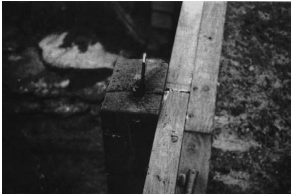
Figure 13-37. - Decay in the end grain of a timber rail post (photo courtesy of Duane Yager, USDA Forest Service).
