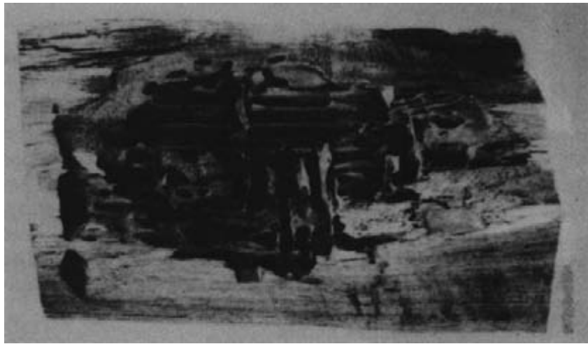
Figure 13-13. - Wood damaged by carpenter ants. The tunnels are generally clear of debris and extend parallel to, and across, the grain.
