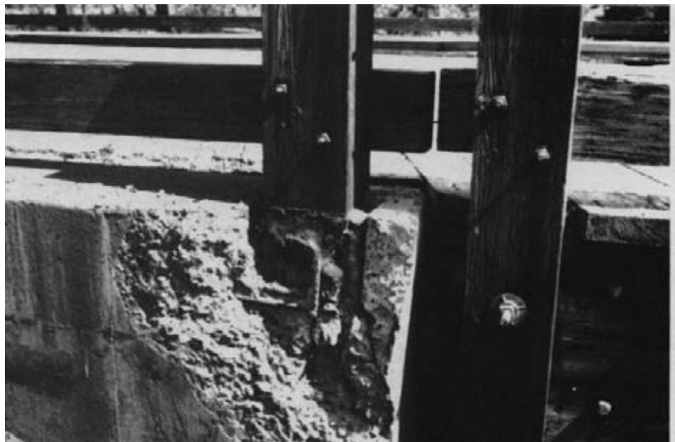
Figure 13-48. - Decay in a timber railpost embedded in concrete at the abutment. Concrete spalling was caused when water trapped in the post cavity was subjected to freeze-thaw cycles.
