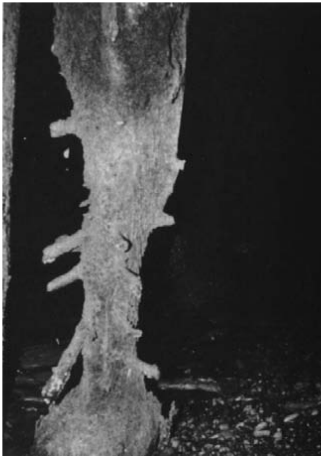
Figure 13-18. - Limnoria damage to a timber pile, evidenced by the characteristic hour-glass shape in the tidalzone.
