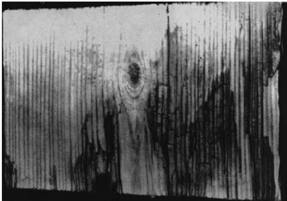
Figure 13-4. - Wood infected with brown rot fungi in an advanced stage. The decayed wood has a darkened color with a cracked, brittle surface that resembles charred wood.
