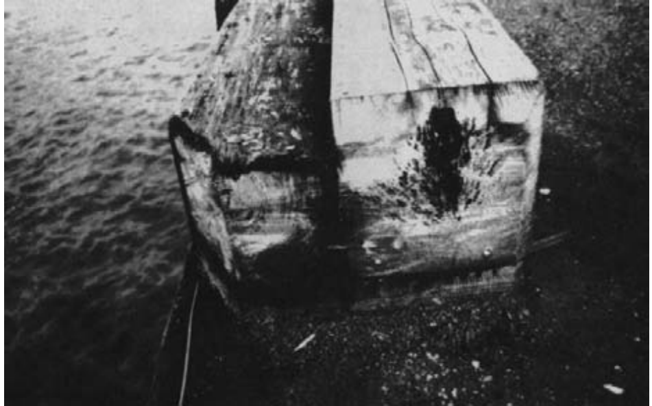
Figure 13-38. - Cross section of a timber curb, exposed by sawing, reveals interior decay resulting from seasoning checks in the upper surface.
