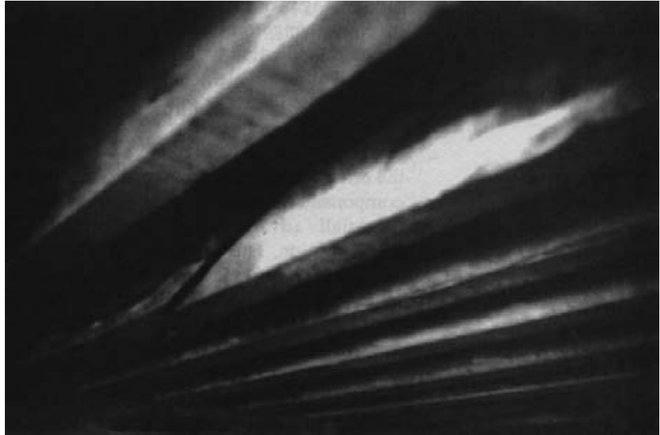
Figure 13-40. - Large crack in a sawn lumber bridge beam caused by vehicle overloads (photo courtesy of Duane Yager, USDA Forest Service).
