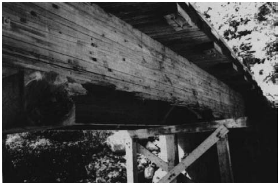
Figure 13-19. - Severe mechanical damage to a glulam bridge caused by debris flow during high stream levels.
