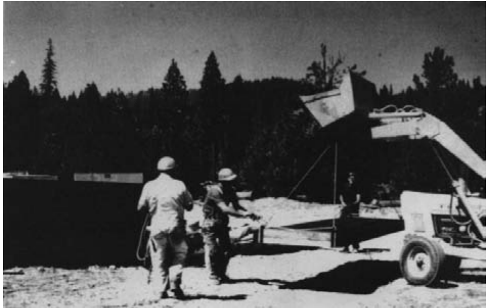
Figure 12-8. - Lifting a glulam deck panel from steel C-brackets that fit over the panel ends.
