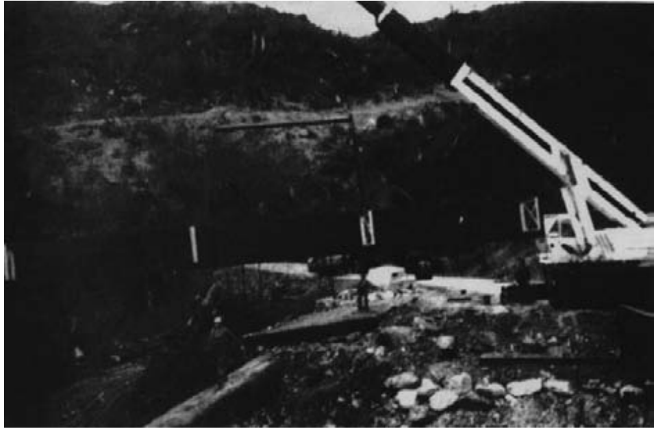
Figure 12-13. - Glulam beam is lifted into position with steel components in place. Note the use of a spreader beam and nylon straps for lifting (photo courtesy of Western Wood Structures, Inc.).
