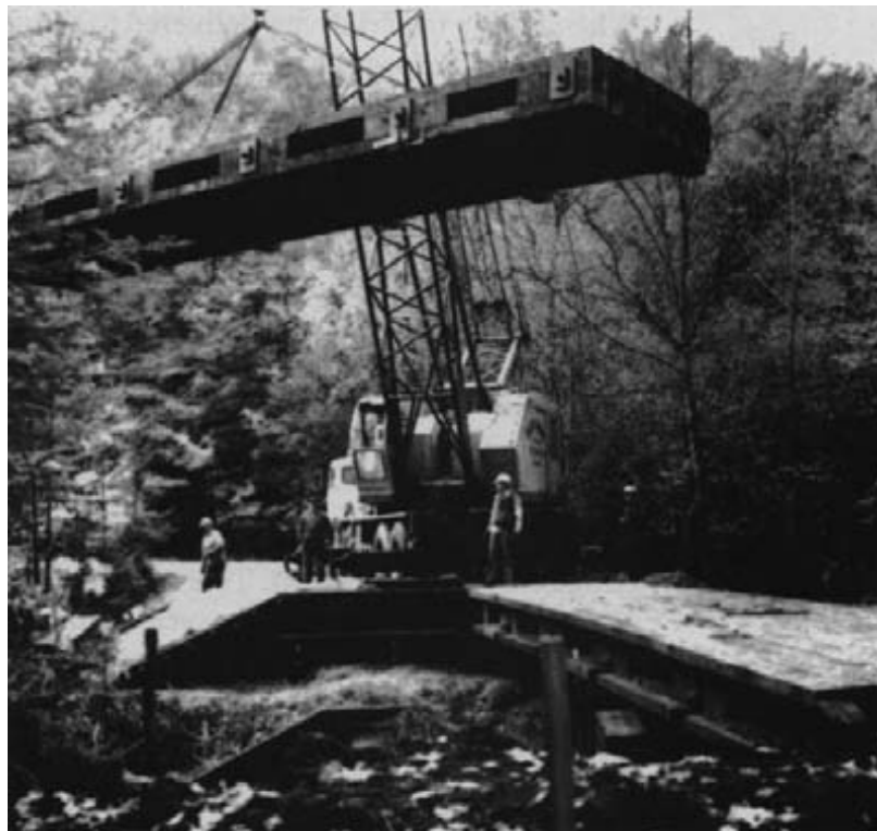
Figure 12-11. - One-half of a stress-laminated parallel-chord bridge is lifted into place by a crane.
