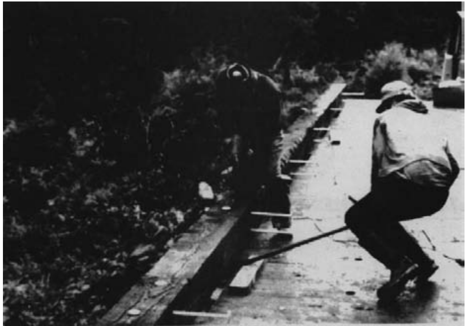
Figure 12-17. - Workers use a pry bar to align the curb for deck attachment.
