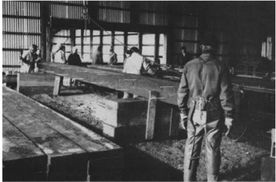
Figure 12-2.- Shop fabrication of timber bridge components, such as these nail-laminated lumber deck panels, is more accurate and more cost effective than field fabrication (photo courtesy of Wheeler Consolidated, Inc.).
