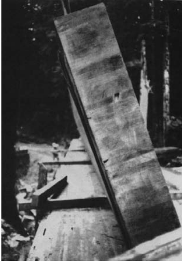
Figure 12-7. - A large glulam bridge beam is tipped from its horizontal storage position before being lifted into place on edge (photo courtesy of Tim Chittenden, USDA Forest Service).
