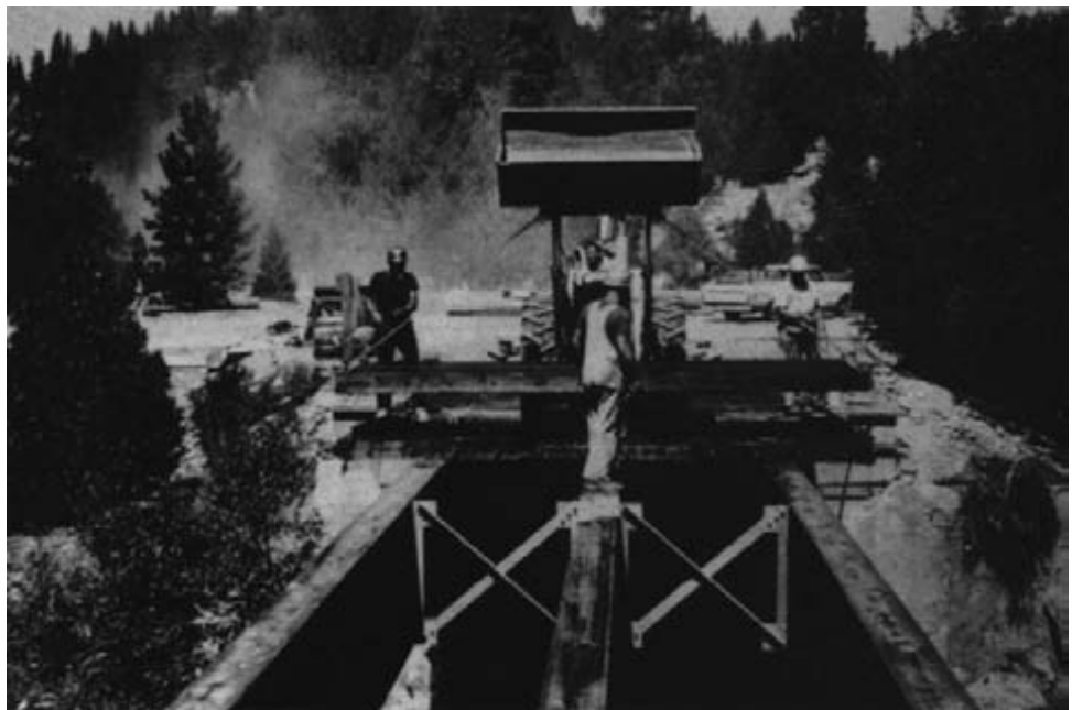
Figure 12-15. - Glulam deck panels are sequentially lifted into place with a backhoe, using C-brackets over the panel ends.
