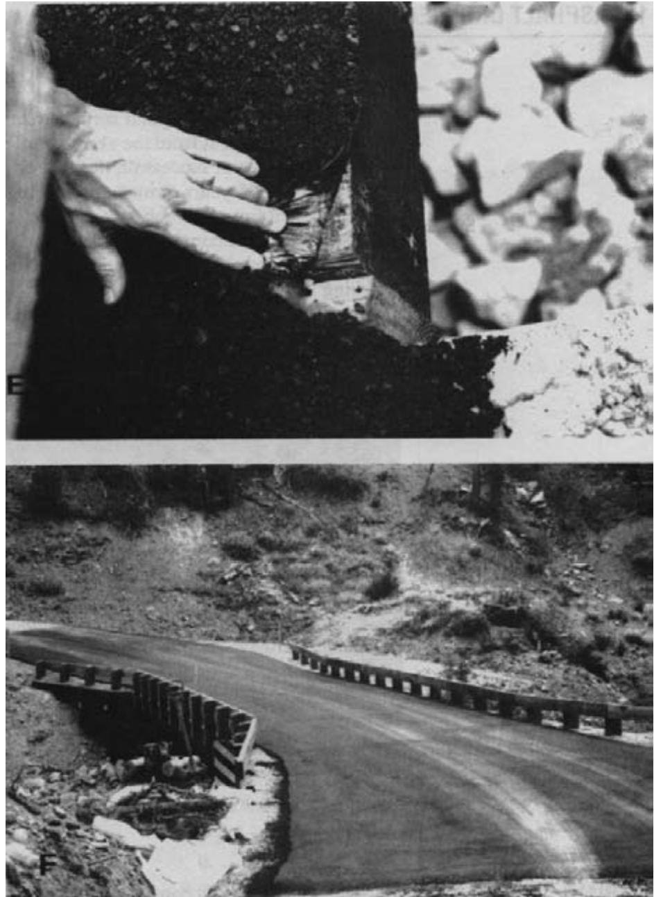
Figure 11-7. - Asphalt paving sequence on a glulam bridge deck using impregnated geotextile fabric (continued). (E) A corner of the fabric is pulled back after application of the hot asphalt, showing the bond between the rubberized asphalt on the fabric and the bridge deck. (F) The completed wearing surface (photos courtesy of Ron Vierra, USDA Forest Service).
