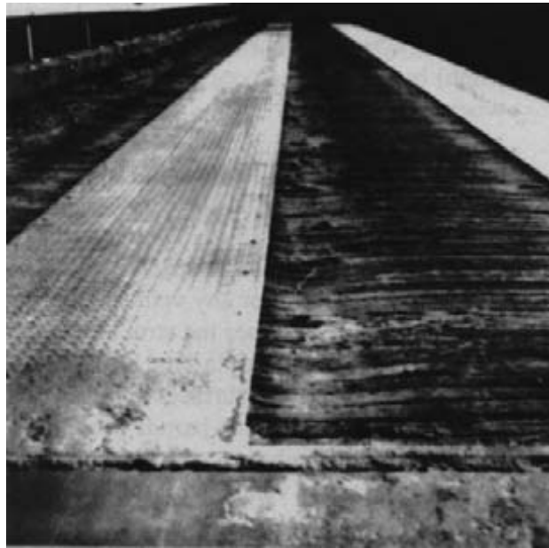
Figure 11-2. - Severe abrasion on a nail-laminated lumber deck caused by vehicles off-tracking the partial steel plate wearing surface (photo courtesy of Sakee Poulakidas, USDA Forest Service).
