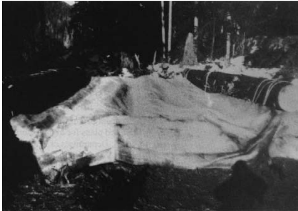
Figure 11-30. - Geotextile fabric placed across a log stringer bridge before placement of an aggregate wearing surface (photo courtesy of Neil Newlun, USDA Forest Service).
