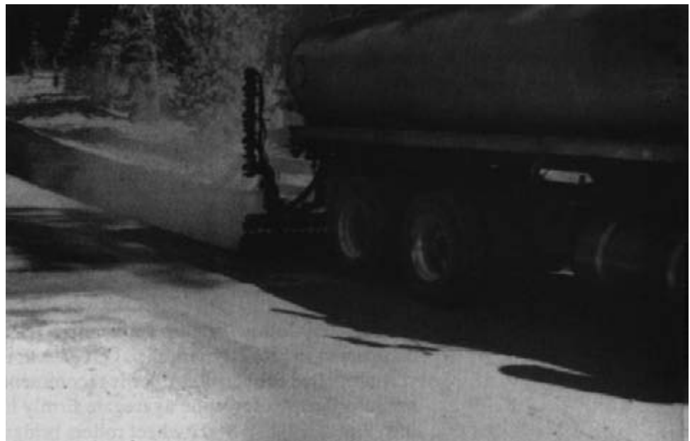
Figure 11-9. - Asphalt binder for a chip seal being applied to a timber bridge deck by an asphalt distributor truck (photo courtesy of Paul Cole, USDA Forest Service).
