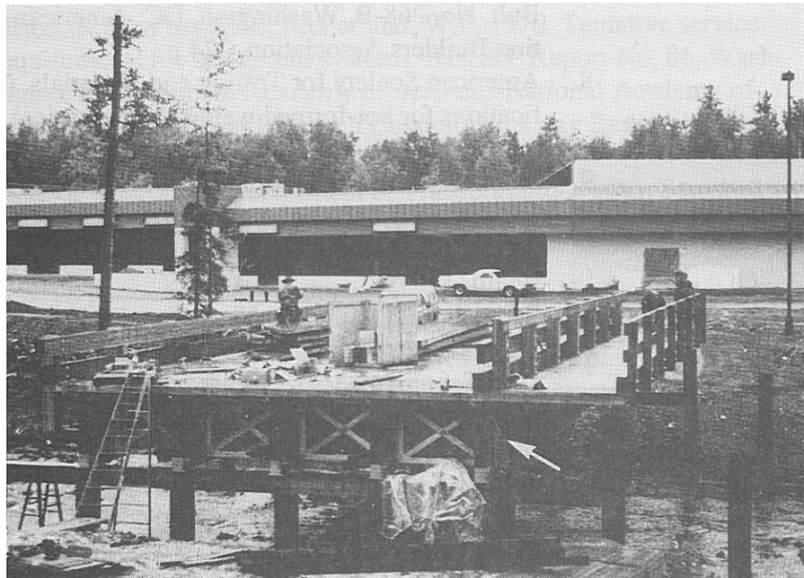
Figure 10-16. - Combination railing posts attached to glulam beams (arrow) through a cutout in the glulam deck (photo courtesy of Western Wood Structures, Inc.).
