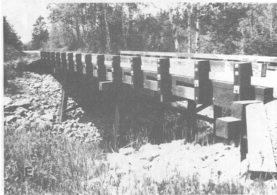
Figure 10-9. - Typical vehicular railing configurations used on timber bridges (continued). (D) Glulam posts and rail with a partial parapet bolted to a glulam deck (photo courtesy of LamFab Wood Structures, inc.). (E) Lumberposts bolted to the lumber curb on a longitudinal nail-laminated lumber deck (photo courtesy of Wheeler Consolidated, Inc.).
