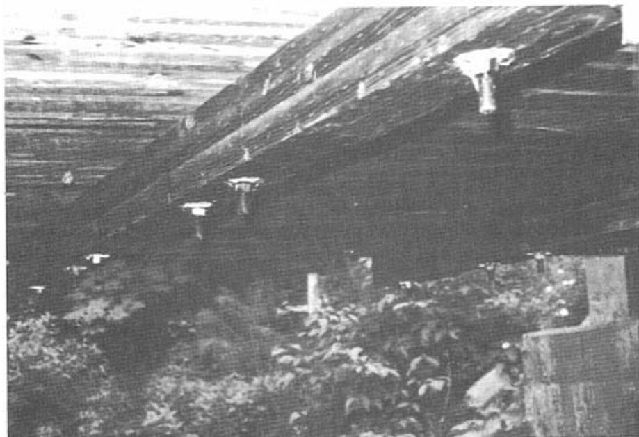
Figure 8-4. - Transverse glulam stiffener beam attached to the underside of a longitudinal glulam deck bridge (photo courtesy of Dave Nordenson, USDA Forest Service).
