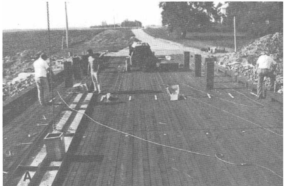
Figure 8-12. - Panelized longitudinal nail-laminated deck bridges. (A) During construction. (photos courtesy of Wheeler Consolidated, Inc.).
