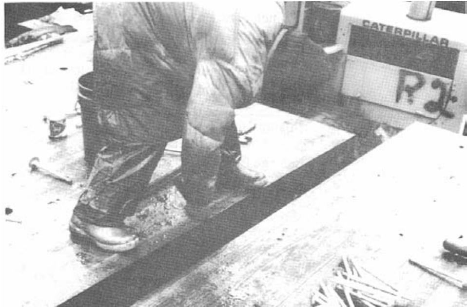
Figure 7-28. - Bituminous sealer is spread on the edges of glulam deck panels to waterproof the panel joints.
