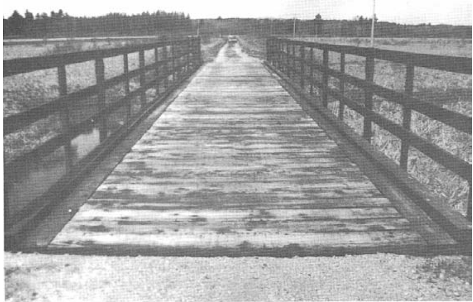
Figure 7-41. - Transverse plank deck on a single-lane, low-volume road (photo courtesy of Wheeler Consolidated, Inc.).
