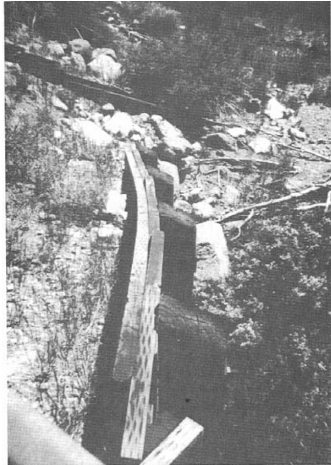
Figure 6-22. - Bulging in an abutment retaining wall caused by earth pressure.
