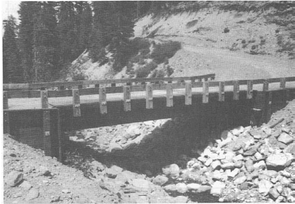
Figure 6-12. - A timber bridge with sharply curved approach roadways. Trucks crossing the bridge can produce centrifugal forces that affect the bridge superstructure and substructure.
