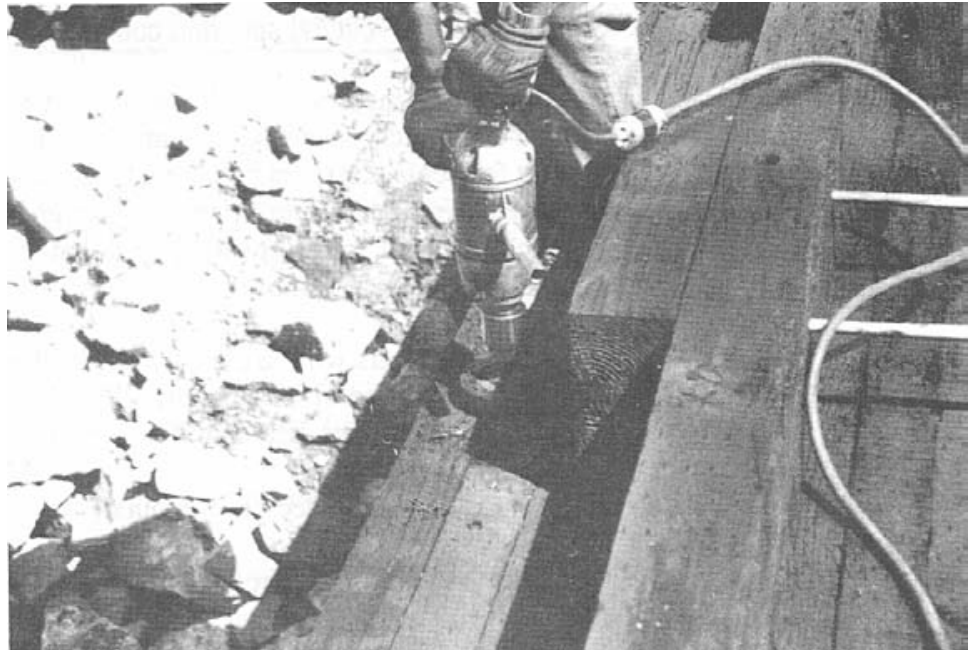
Figure 5-31. - Field-grooving for a split ring connector for a curb-deck attachment. Field fabrication such as this requires field treating with wood preservative, as discussed in Chapter 12 (photo courtesy of Wheeler Consolidated, Inc.).
