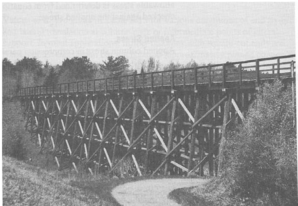
Figure 5-7.- Timber columns are common in bridge substructures such as these bents (photo courtesy Wheeler Consolidated, Inc.).
