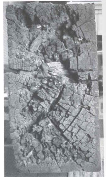
Figure 1. — Beam with extensive decay at end.
